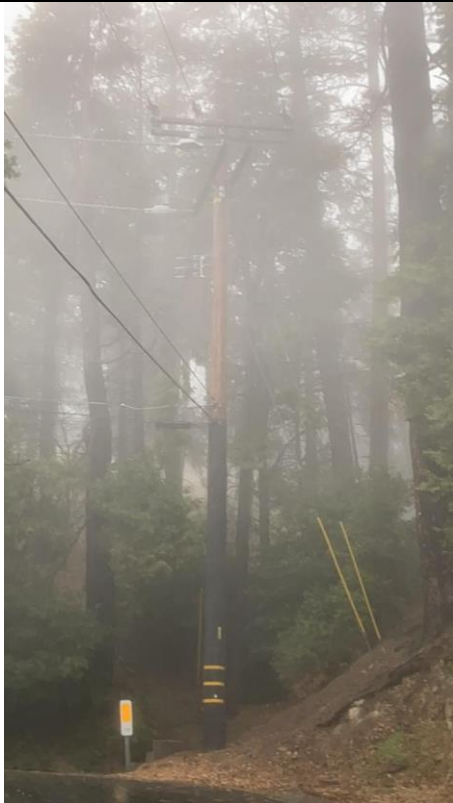
Item8GImg1: Overall pole
