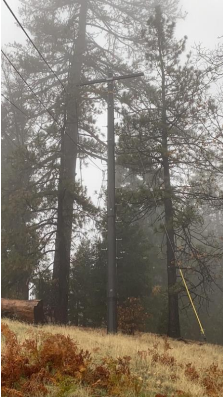
Item10GImg1: Overall pole
