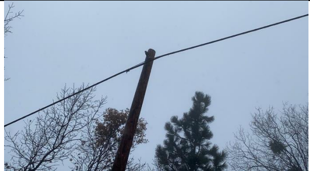
Item9IA1Img2: Zoomed out view of top of pole with no covered conductor
