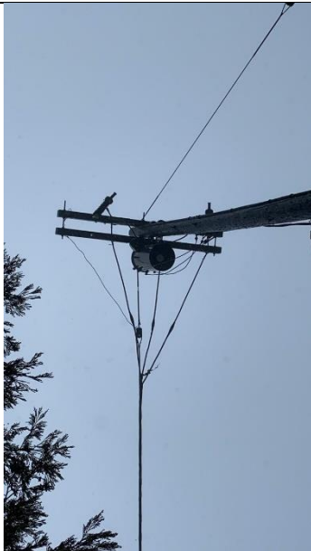
Item11IA1img1: No covered conductor installed
