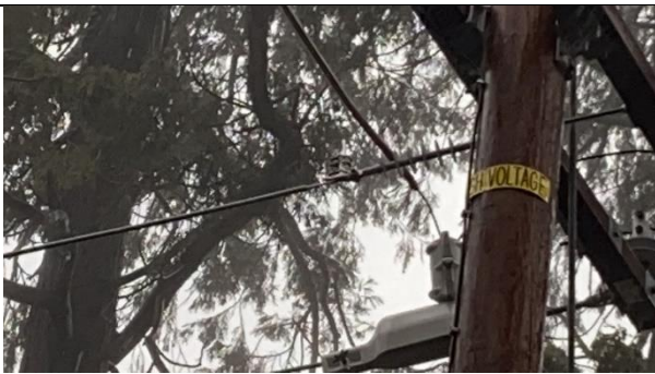
Item3IA4Img1: Bare dead-end conductor with no cover
