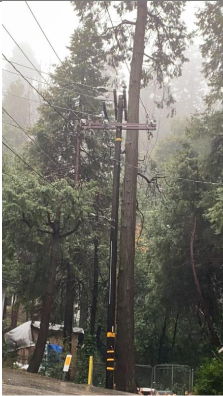
Item4GImg1: Overall pole
