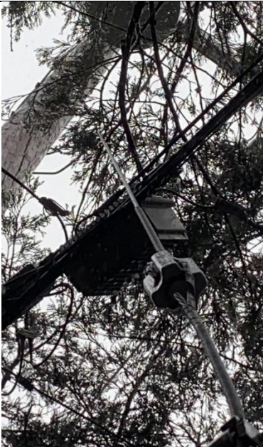
Item7GW21mg1: Vegetation touching guy wire above insulator
