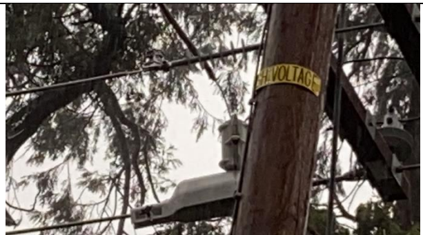
Item3IA5Img2: Overall photo bare jumper going into bolted wedge connector cover
