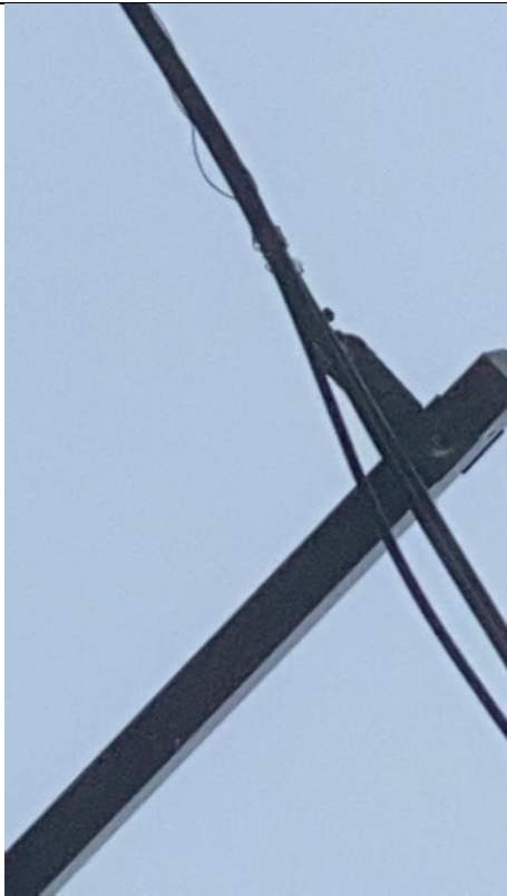
Item10CD4Img1: Fraying conductor
