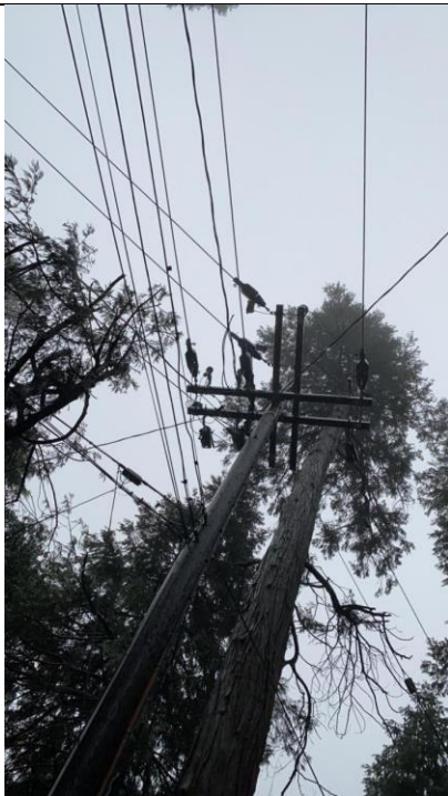
Item4IA1Img1: No vibration dampers
