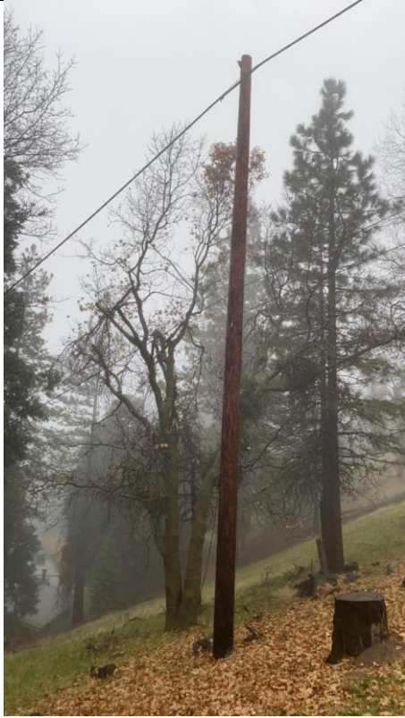
Item9GImg1: Overall pole
