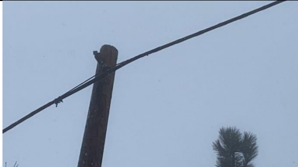
Item9IA1Img1: Close up no covered conductor
