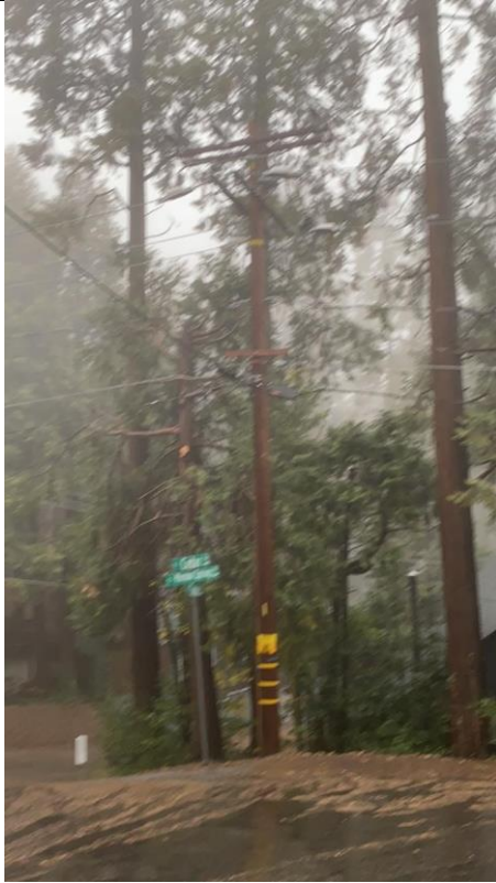
Item3GImg1: Overall pole
