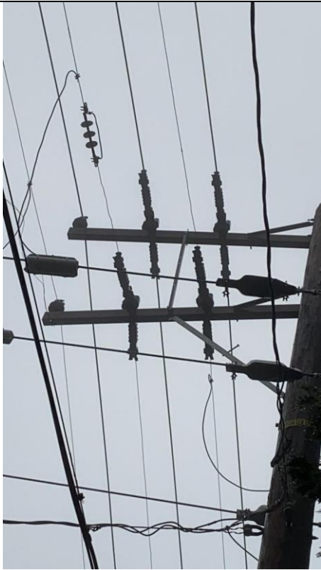
Item1IA1Img1: Top level crossing phase showing bare wire and no covered conductor installed
