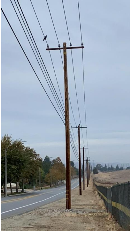
Item8GImg1: Overall pole
