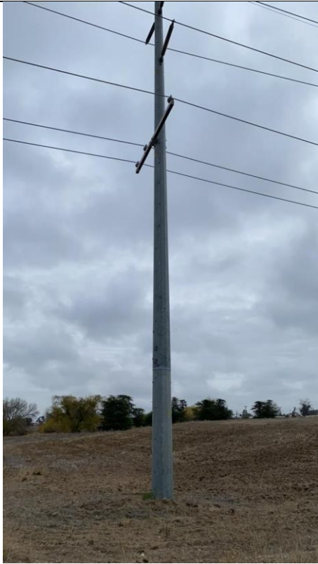
Item17G1mg1: Overall pole
