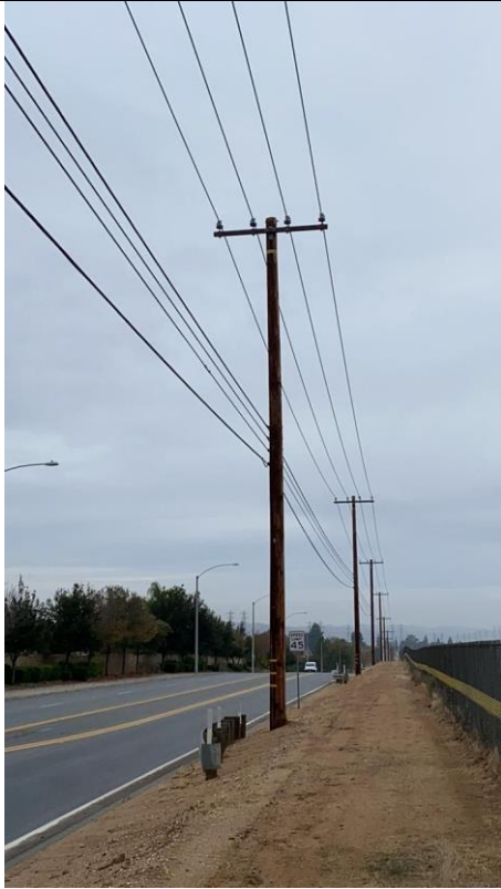
Item5Gimg1: Overall pole
