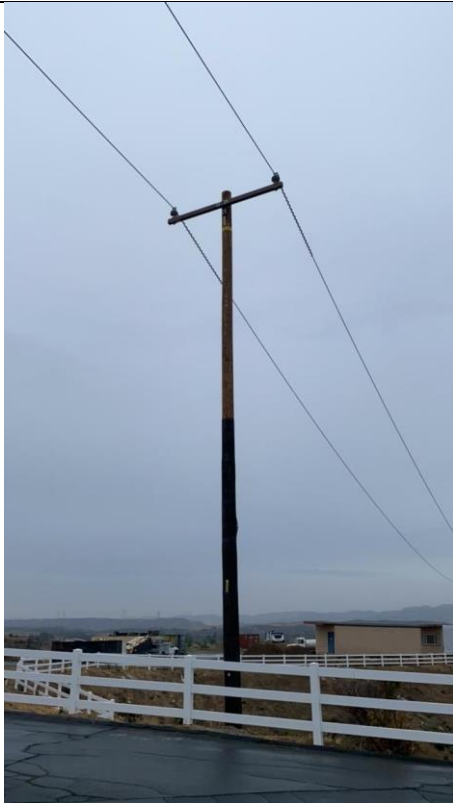
Item2GImg1: Overall pole
