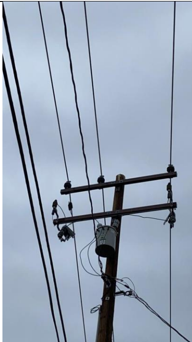
Item15IA1Img1: No vibration dampers
