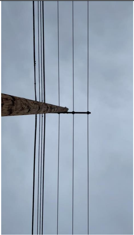
Item7IA1Img1: No vibration dampers
