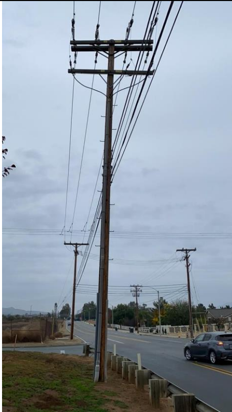
Item3GImg1: Overall pole
