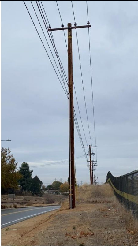
Item11Gimg1: Overall pole
