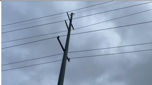
Item17IA1mg1: No vibration dampers
