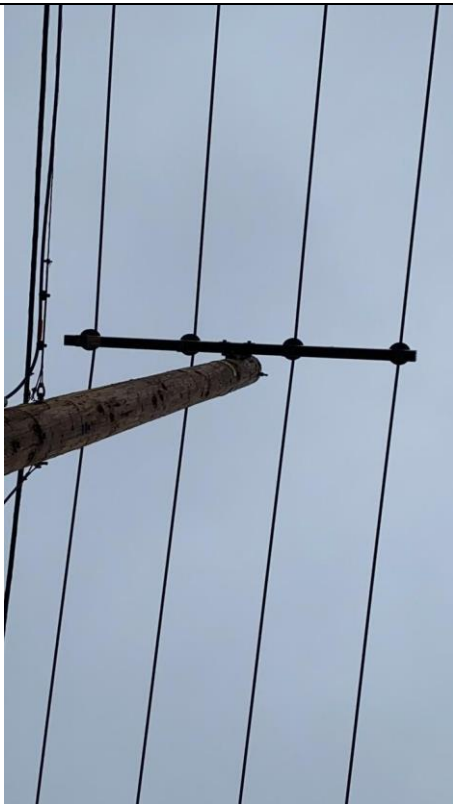
Item11IA1mg1: No vibration dampers
