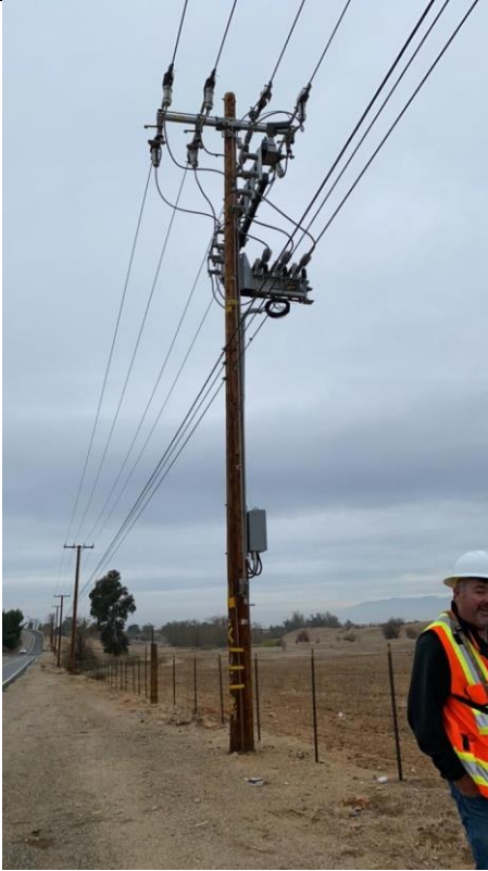
Item13G1mg1: Overall pole
