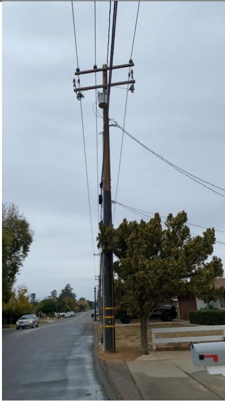
Item15GImg1: Overall pole
