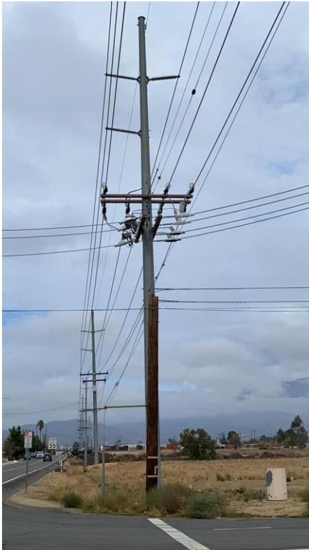
Item16G1mg1: Overall pole
