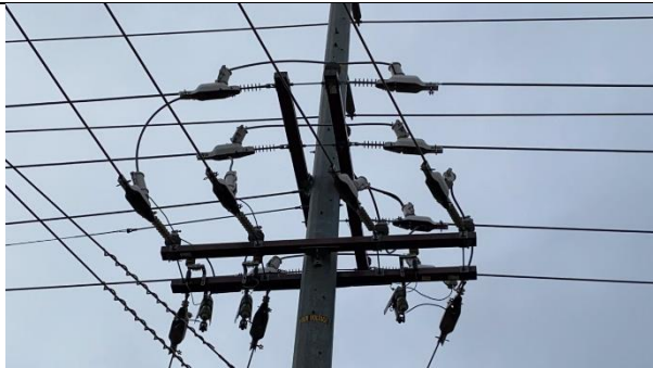
Item16IA2img1: No vibration dampers
