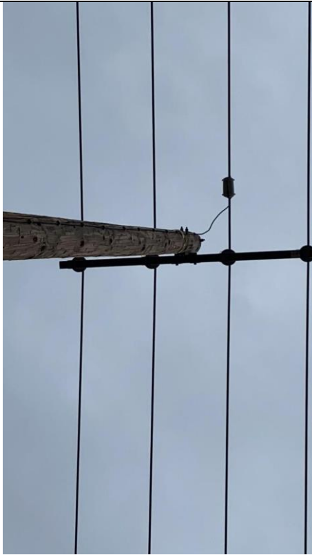
Item6IA1Img1: No vibration dampers
