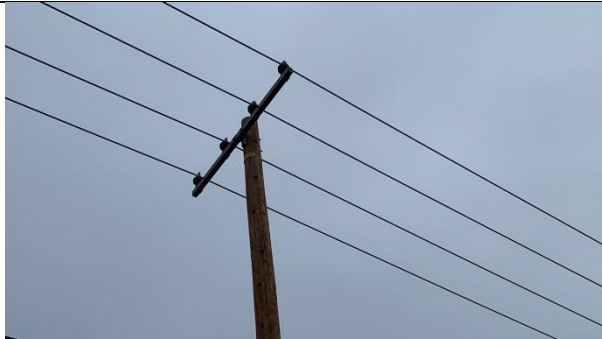
Item4IA1img1: No vibration dampers
