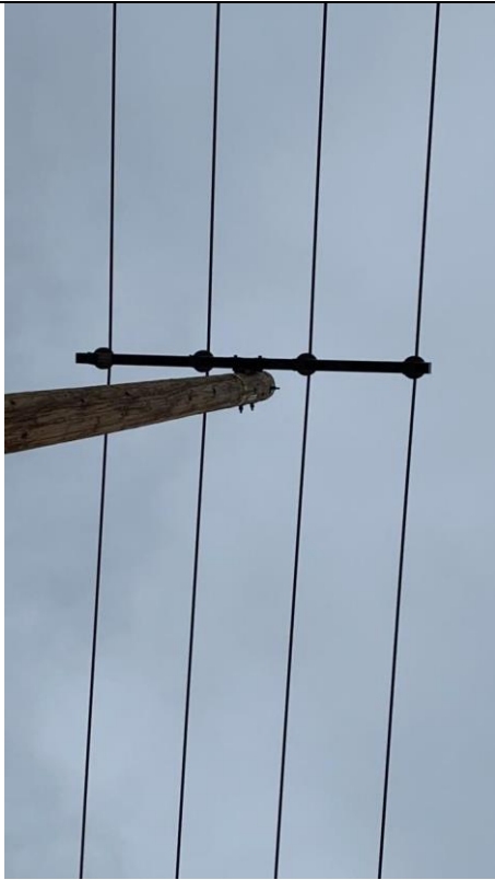
Item10IA1mg1: No vibration dampers
