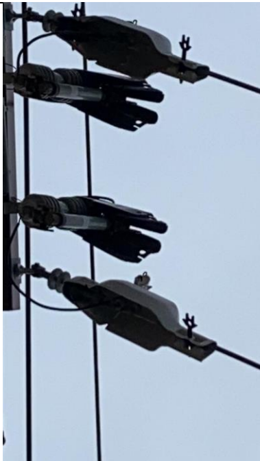
Item16IA4Img1: Loose dead-end clamp
