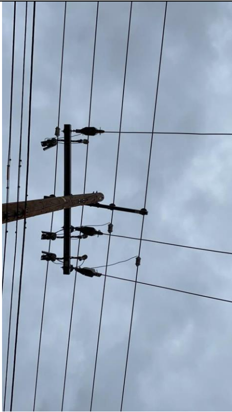
Item12IA1Img1: No vibration dampers
