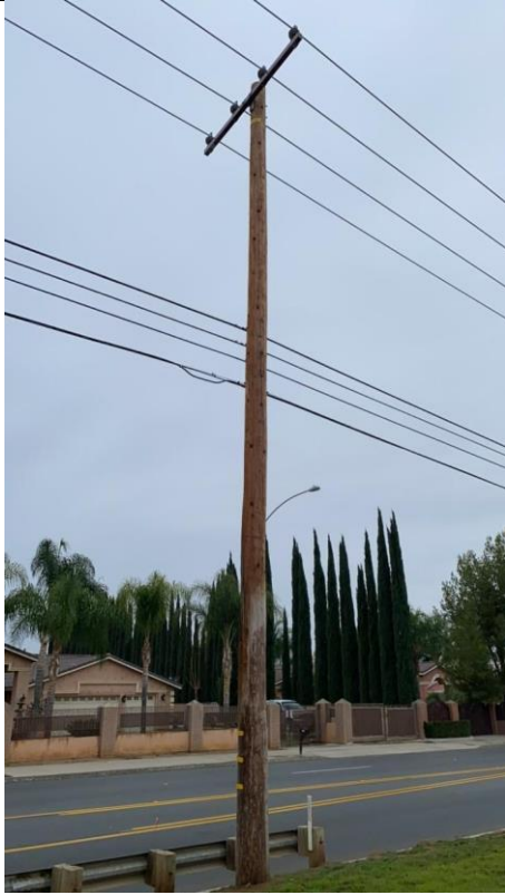
Item4Gimg1: Overall pole
