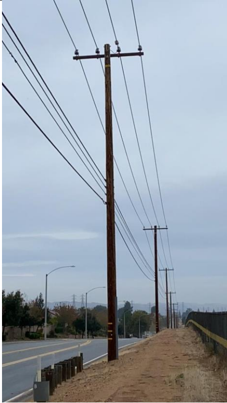
Item6GImg1: Overall pole
