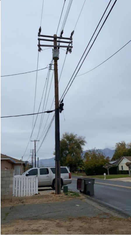
Item14GImg1: Overall pole
