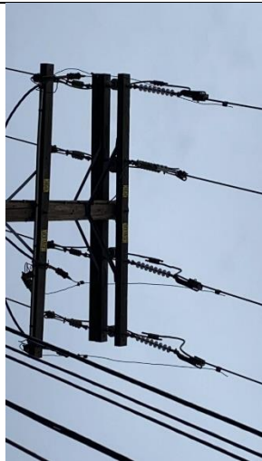
Item3IA1img1: Bare conductor when data indicates that there should be covered conductor
