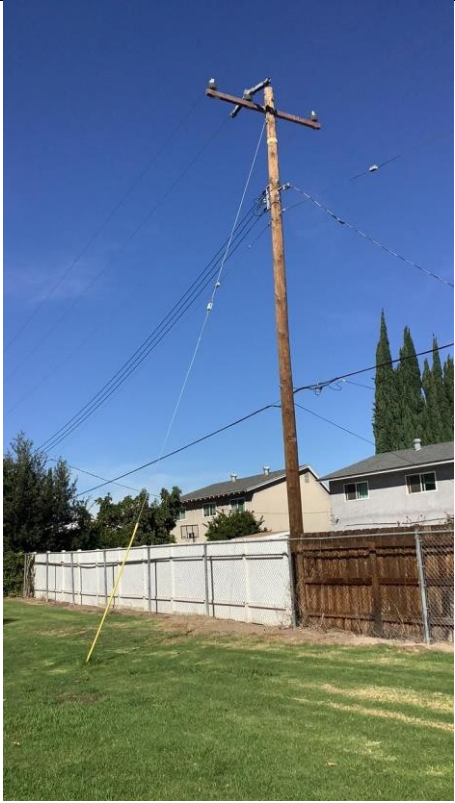
Item6GW1Img1: Overall view of loose guy wire
