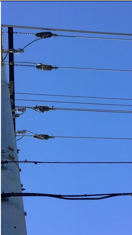
Item1IA1img1: At dead end, no vibration dampeners installed
