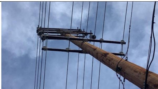
Item4IA1img1: Vibration dampers not installed
