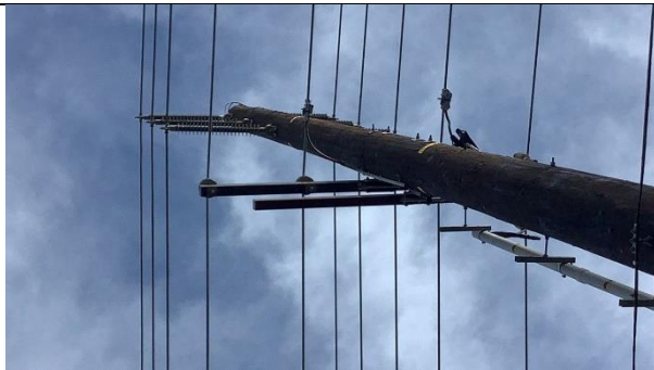
Item5IA1Img1: Vibration dampers not installed
