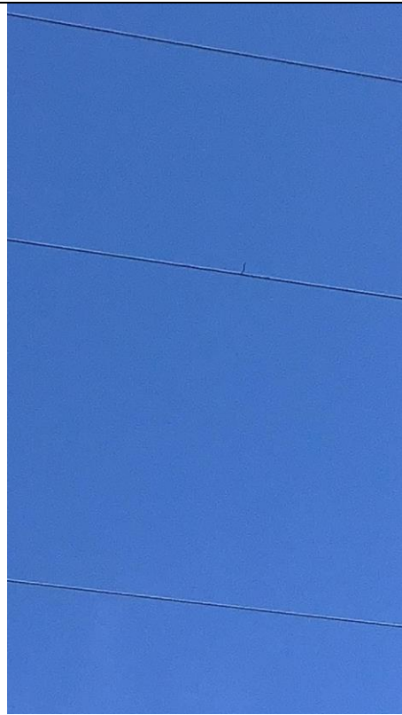
Item7CD4Img2: Close up of frayed conductor
