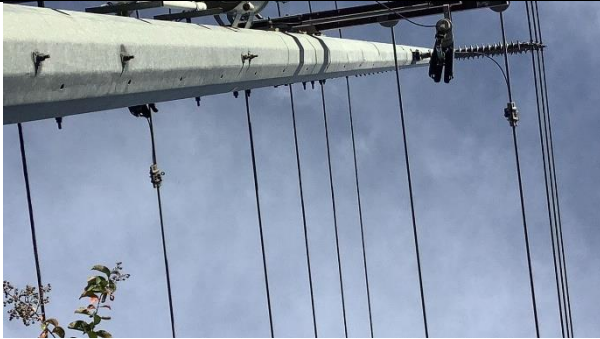
Item8IA1Img3: No vibration dampers installed
