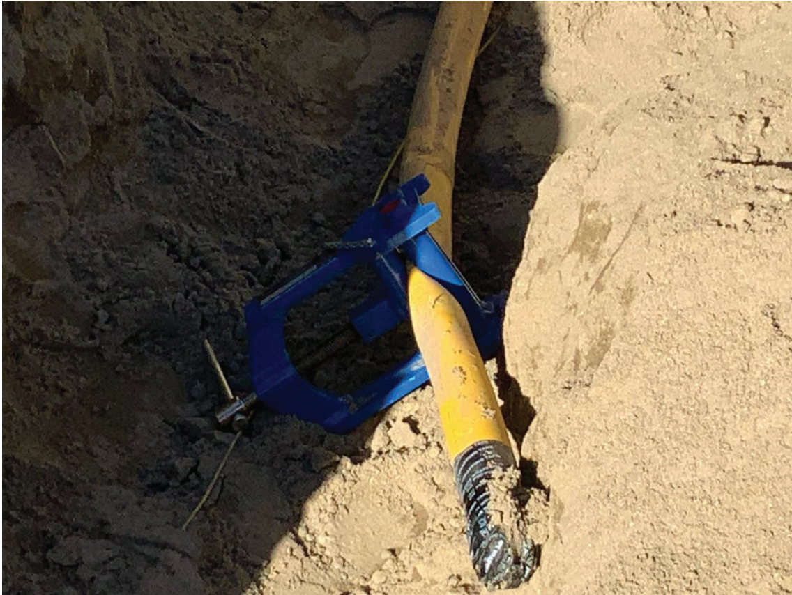
Photo 2 – Gas Line Pinched by Contractor (Photo provided by SoCal Gas)
