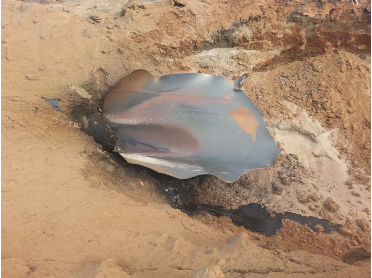
Figure 4. A photograph of the downstream pipe at the rupture location.
