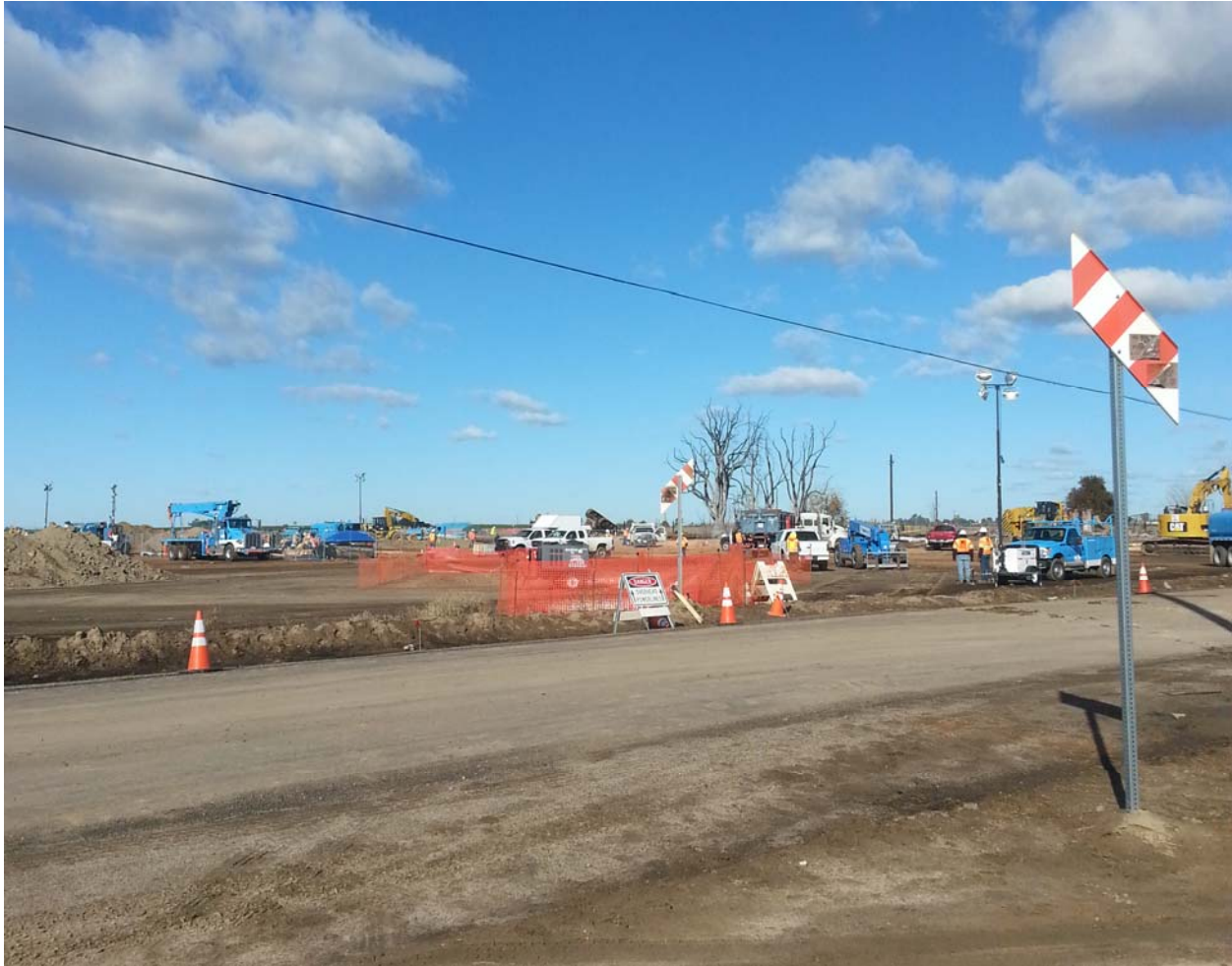
Figure 6. A photograph of pipeline markers upstream of the strike location.
