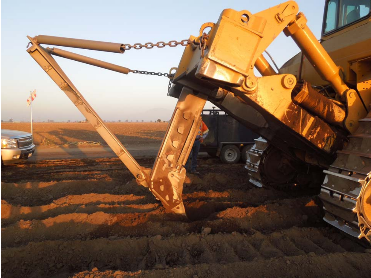
Figure 1. A photograph of the D10 Caterpillar with the 6 foot ripper attachment near the strike location. A PG&E line marker can be seen in the background.
