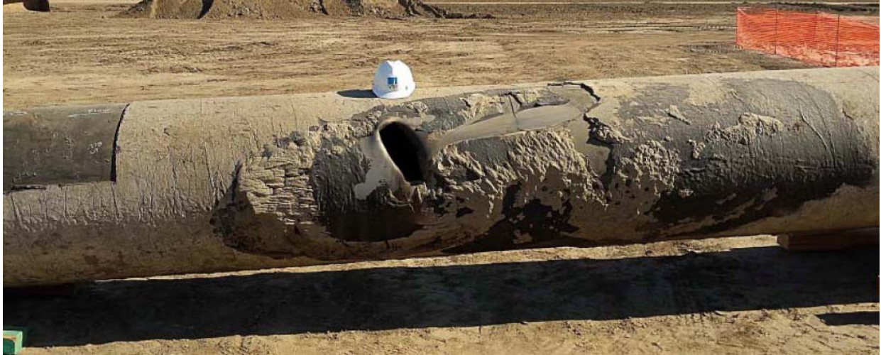
Figure 2. A photograph of the 100% through-wall puncture on L-300A – gas flow from right to left.
