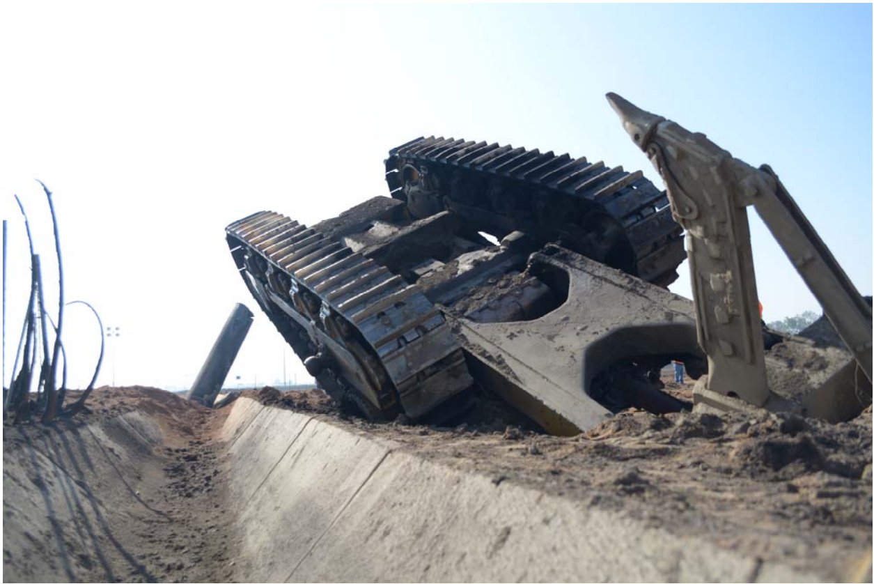
Figure 5. A photograph of the overturned tractor with the ripper blade. Geotechnical analysis indicated the ripper was likely operating at a depth ranging from approximately 60.2 to 63.9 inches. 5
