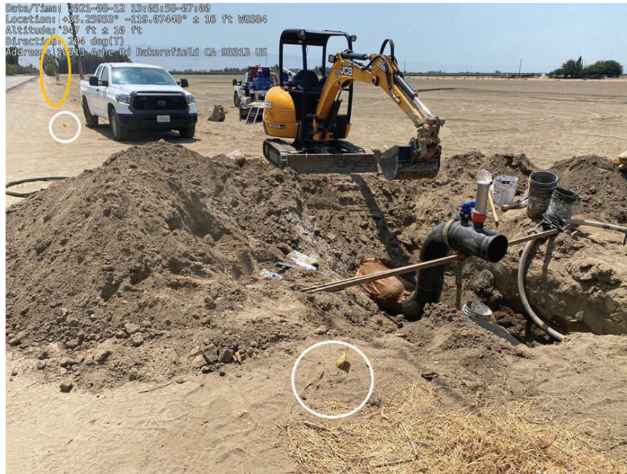
Figure 3: From Exhibit 1, image of excavation area, with diagonal permanent pipeline marker visible next to the second utility pole in the distance (top left of photo). Photo from Crimson Pipeline. White circles and orange oval added for clarity.
