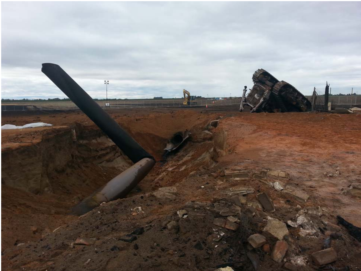
Figure 2. A photograph of PG&E Line 300A at the strike location. The overturned tractor involved in the incident can be seen in the background.
