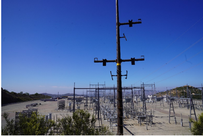
327 500/230-kV substation, 1 steel riser pole (empty), View S
