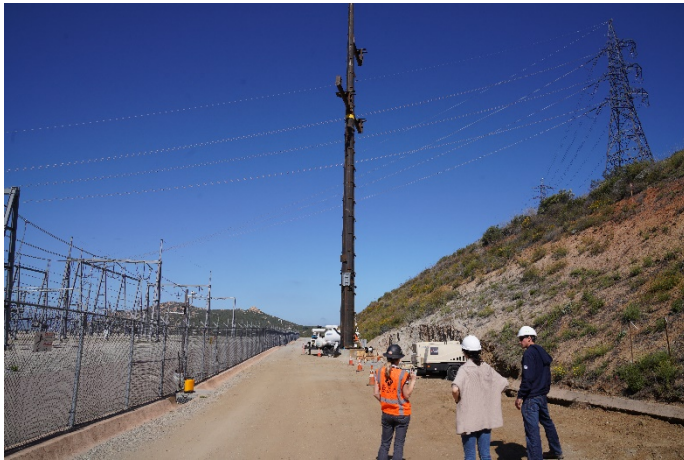
339 500/230-kV substation, 1 steel riser pole (empty), View S
