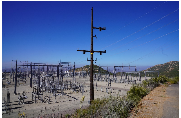
320 500/230-kV substation, 1 steel riser pole (empty), View S
