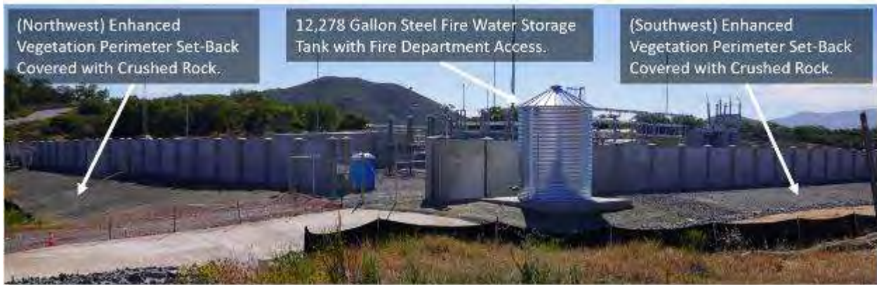
Figure 4. Fire Dept. Water Tank, NW Corner
