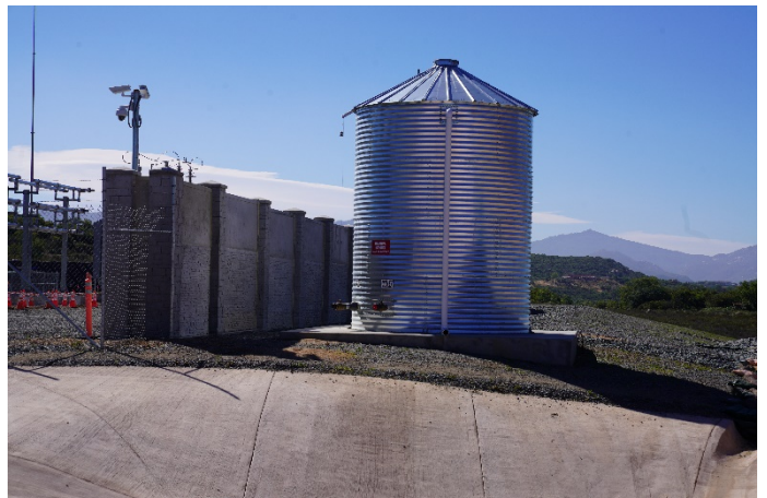
306 Fire Dept. Water Tank, NW corner, Exterior, 12,278 gal
