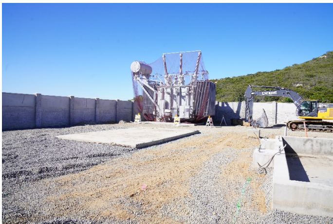
272 Spare Tx under netting (500-kV) View Southwest
