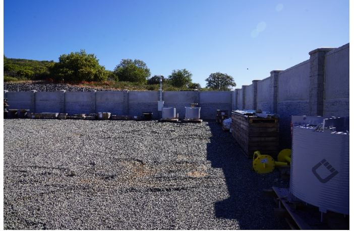
281 Capacitor bank reactors, View North
