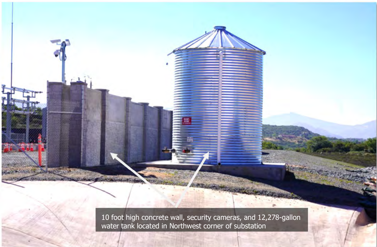
Figure 10. Fire Dept. Water Tank, NW Corner, Exterior, 12,278 gal
