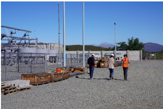
284 Reactors, Control Building, View North
