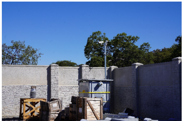
291 Cameras, Interior Northeast corner
