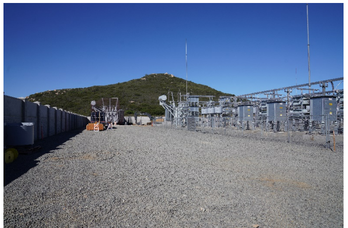
285 Tx, Reactors, Resistors, View West, Wide view
