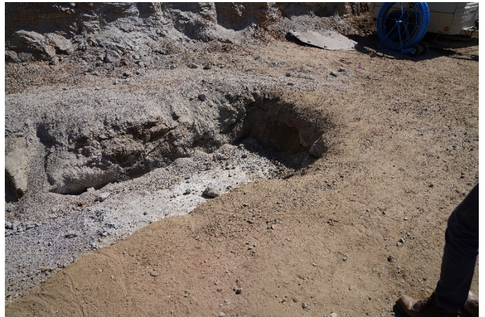
343 Hole in ground, top of concrete encased duct bank
