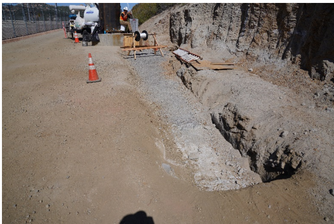
344 Steel riser pole base with worker installing pull cord in conduit, concrete covered trench
