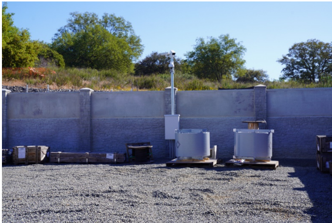
282 Cameras, reactors, View South, close up
