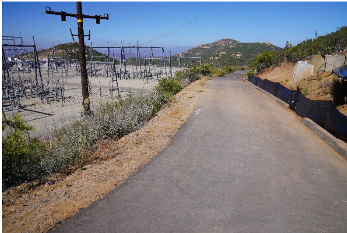
331 1 steel riser pole (empty), View South
