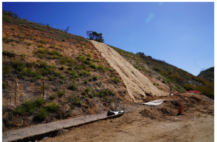
345 material covering washout on hill, View Northeast
