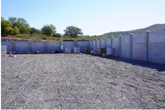
274 Capacitor bank reactors, View North
