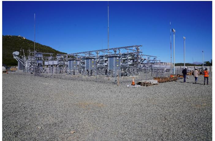
283 Tx, Reactors, Resistors, View Northwest
