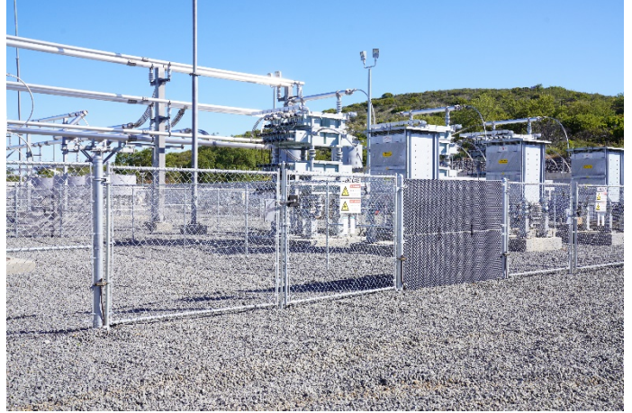
275 Capacitor banks, View North
