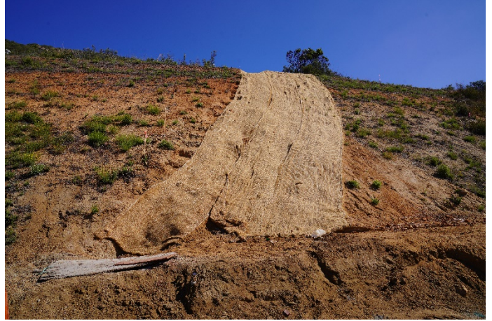
338 material covering washout on hill, View North
