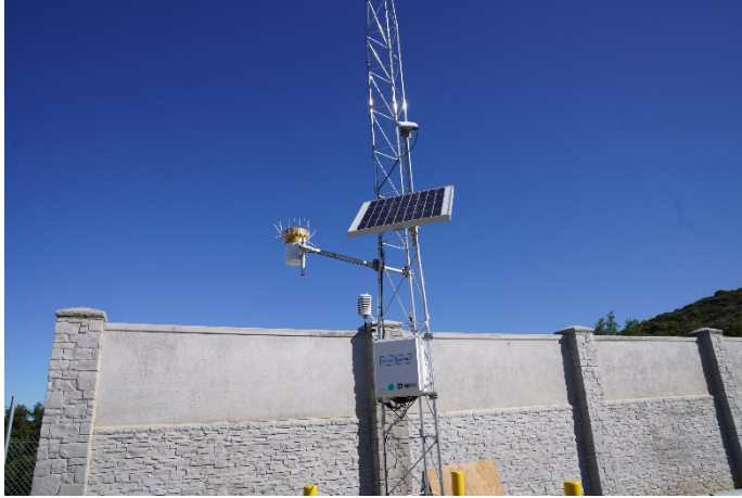
268 Weather Station, Exterior, View North
