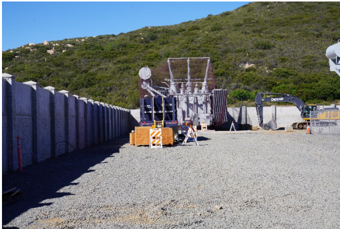
286 Denbeste trailer, Spare Tx, View West
