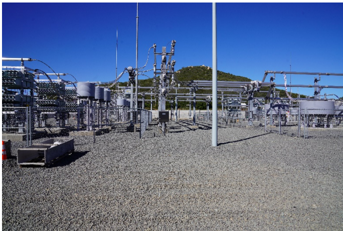
288 Capacitor banks & Reactors, Reactors
