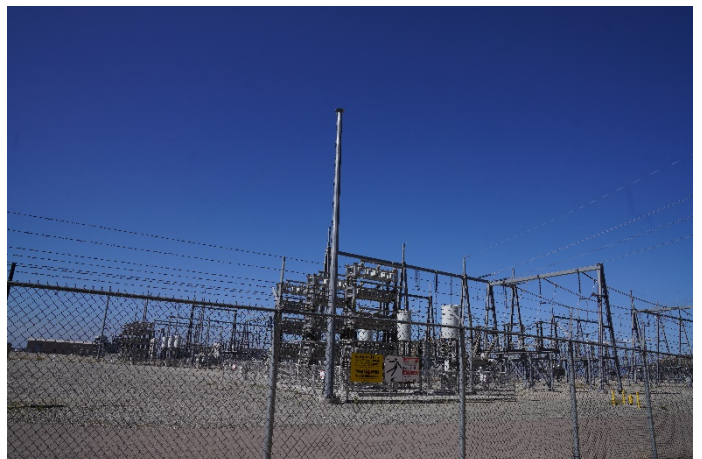
336 500/230-kV substation, View Southwest
