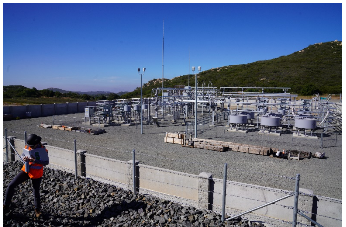
297 Reactors, Capacitor banks, Elevated view West
