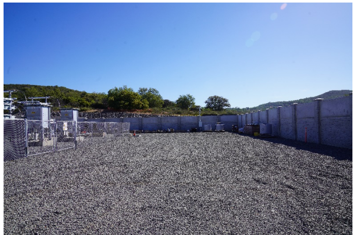
277 Capacitors Reactors, View South, Wide view
