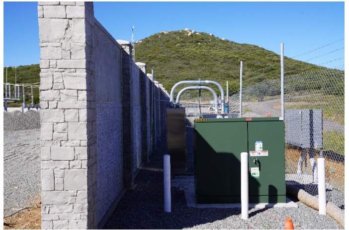
295 North Wall, Exterior, Station transformers, View West
