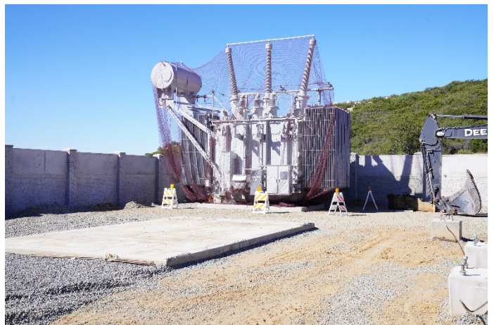
273 Spare Tx under netting (500-kV) View Southwest, close up
