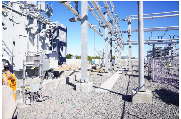
271 Transformer and Capacitors banks, View Northwest
