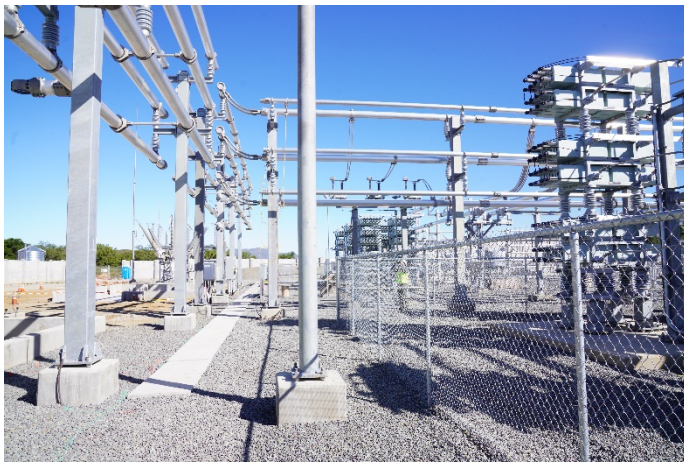
270 Capacitor banks, View Northwest
