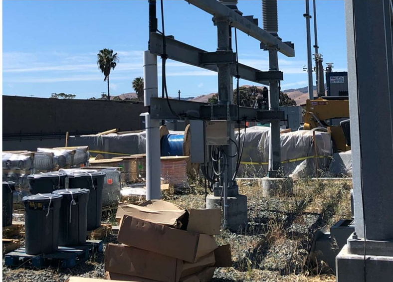
Figure 5. Grass growing within Facility
