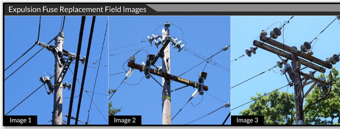
Figure 6: Example Expulsion Fuse Replacement Field Images
