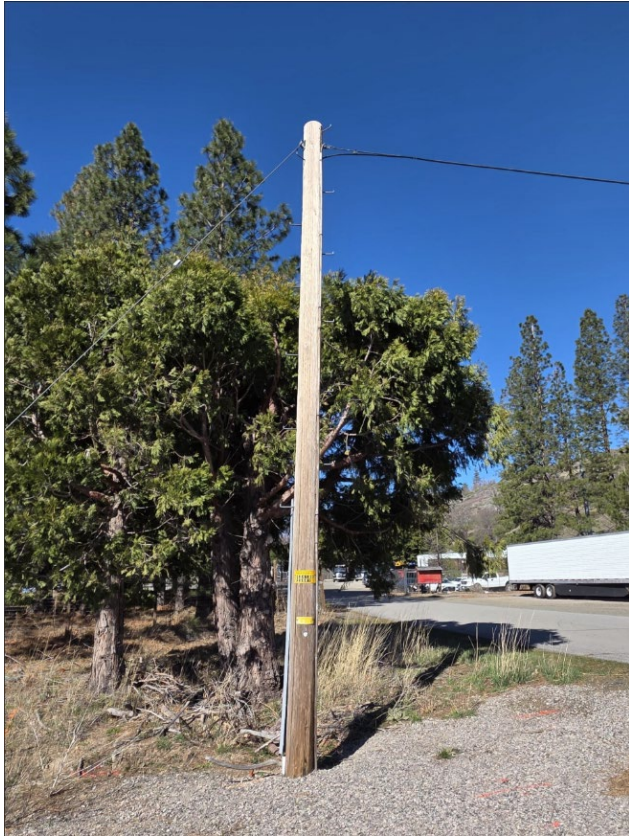
Picture 3: Near Pole ID 06241005.025601, Grid Hardening ID 8077661 at coordinates 41.430728439176896, -122.38954876481279. Picture taken March 6, 2026.
