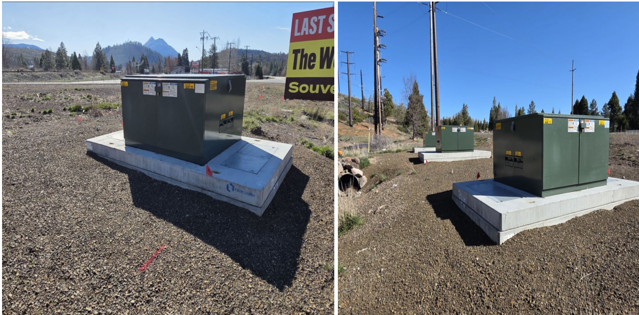
Pictures 1-2: Near Pole ID 06241005.026663, Grid Hardening ID 8077661s at coordinates 41.4315635714616, -122.388955. Picture taken March 6, 2026.
