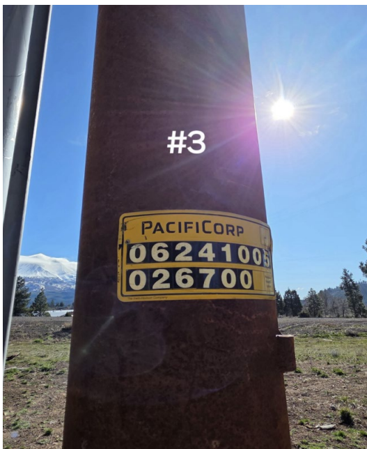
Picture 3: Near Pole ID 06241005.026700, Grid Hardening ID 8077661s at coordinates 41.4315635714616, -122.388970. Picture taken March 6, 2026.
