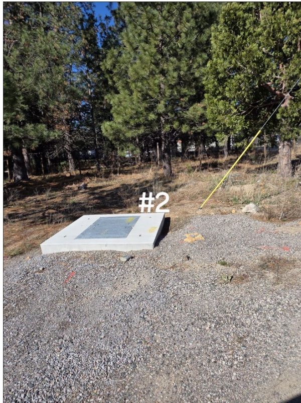
Picture 1: Near Pole ID 06241005.026600, Grid Hardening ID 8077661v at coordinates 41.430785127256, -122.388902. Picture taken March 06, 2026.
