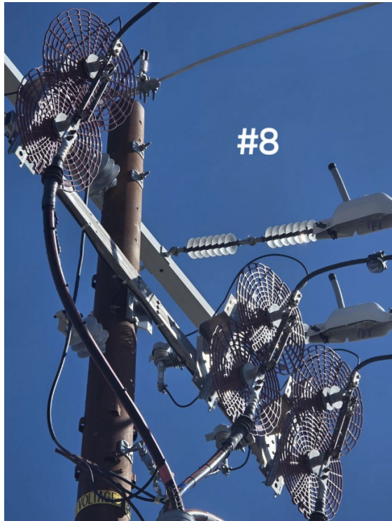
Picture 1: Near Pole ID 06241005.026600, Grid Hardening ID 8077661 at coordinates 41.4293338392048, -122.388872. Picture taken March 6, 2026.
