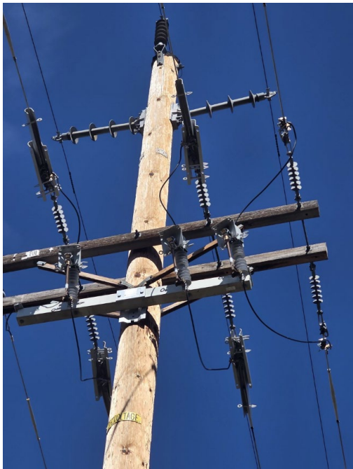
Picture 1: Near Pole ID 20/7X, Grid Hardening ID 7112939 at coordinates 41.7383054840344, -122.615714. Picture taken March 6, 2026.
