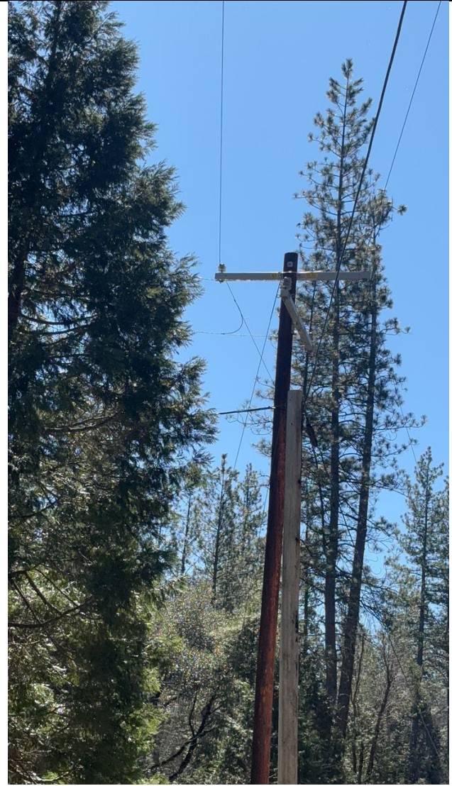
Photo 4: Additional photo of the same cedar tree encroaching within the four-foot minimum clearance distance from the primary conductor. Photo taken north of the tree and pole looking south.
