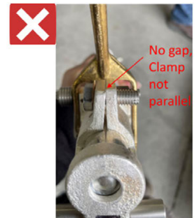
Figure 19 Improper End Fitting Installation
