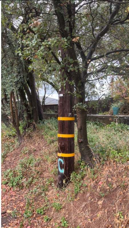
IA1mg2: Vegetation within 10 ft of the base of the pole
