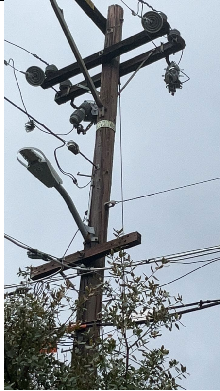
G1mg4: Solid Blade Disconnects and lack of reclosers, sectionalizers, or voltage regulators
