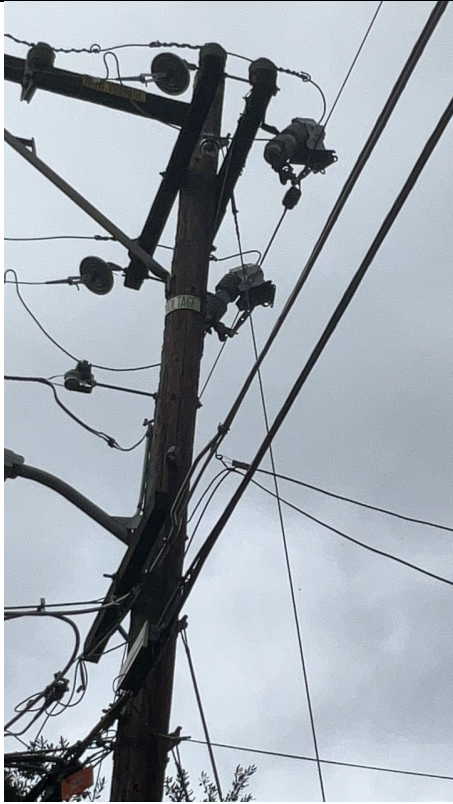
G1mg3: Solid Blade Disconnects and lack of reclosers, sectionalizers, or voltage regulators
