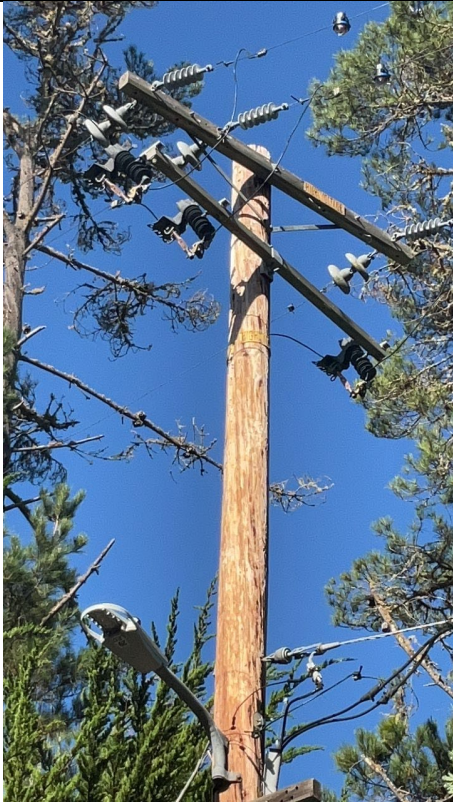
IA1Img2: Solid blade disconnects without reclosers, sectionalizers, or voltage regulators also on the pole.
