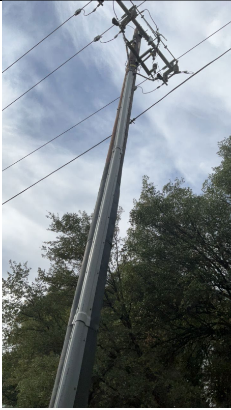
IA1Img3: Riser at the pole, no covered conductor installed east of Pole 121883227
