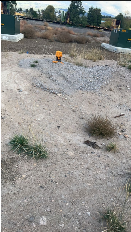
IA1mg2: No CAL FIRE-approved non expulsion fuses at this location
