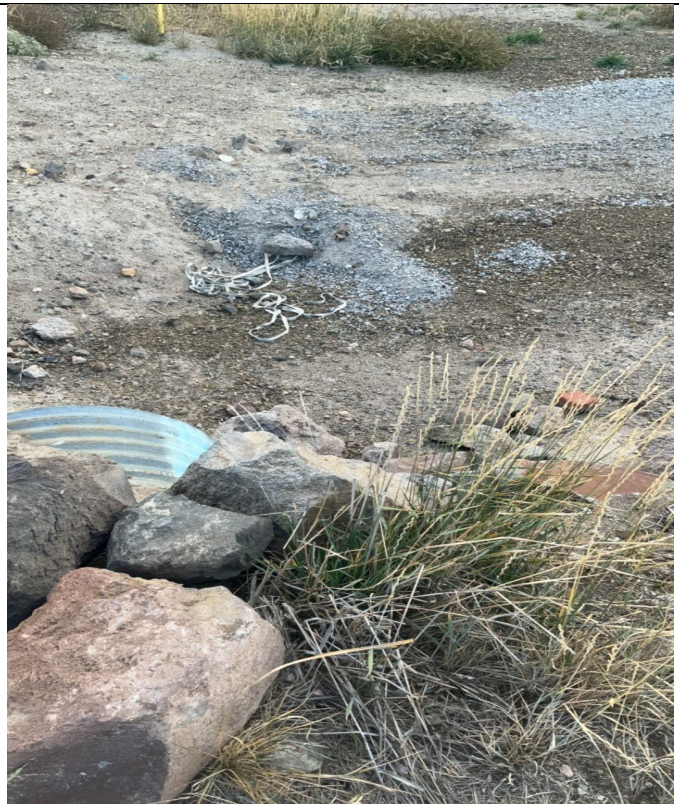
IA1mg3: No sign of CAL FIRE-approved non expulsion fuses at this location
