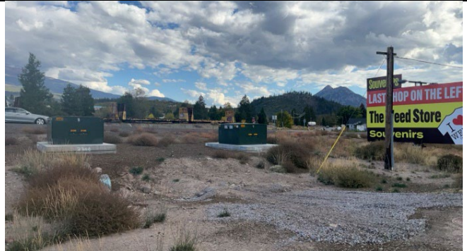
IA1mg1: No sign of CAL FIRE-approved non expulsion fuses at this location
