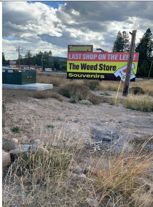
IA1mg2: No sign of CAL FIRE-approved non expulsion fuses at this location
