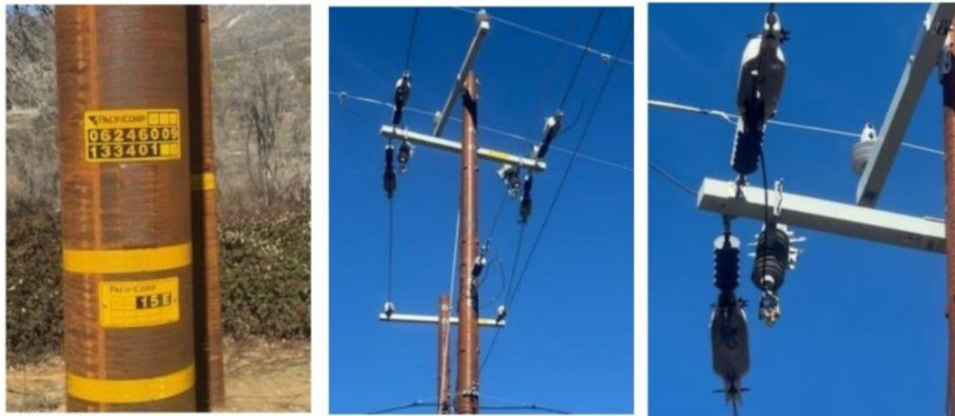
Picture: Near Pole ID 06246009.133401, Grid Hardening ID 7011447i at coordinates 41.83017052263573, -122.8464202100858. Picture taken February 04, 2026.
