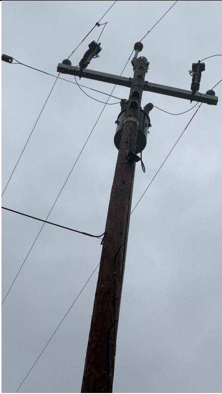
IA1Img3: Close up view of pole 121471467 showing bare conductor on either side
