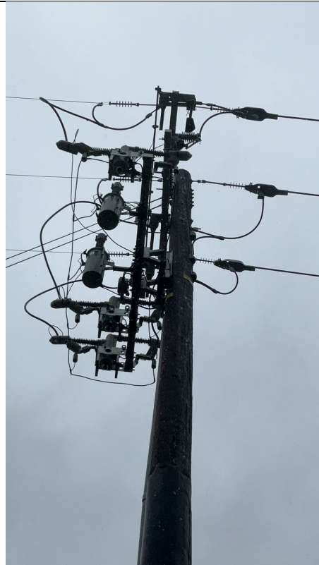
IA1mg2: Close up view of pole 121774370 showing bare conductor on southeast side (Recloser side)
