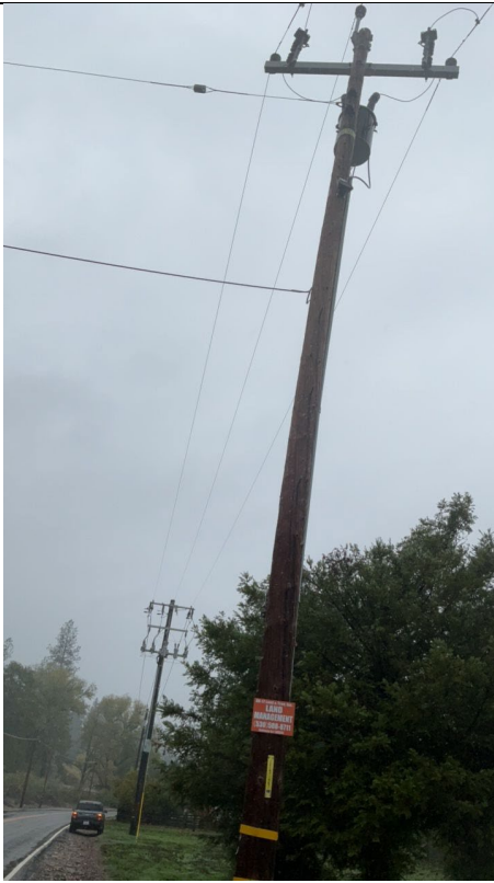
G1mg3: Overall Structure, Northwest-facing view with no covered conductor installed northwest of Pole 121471467
