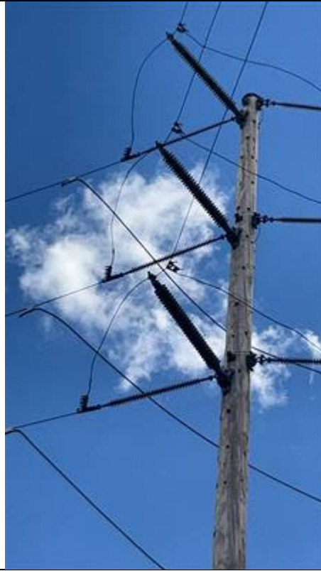
IA1mg2: No covered conductor installed at this location
