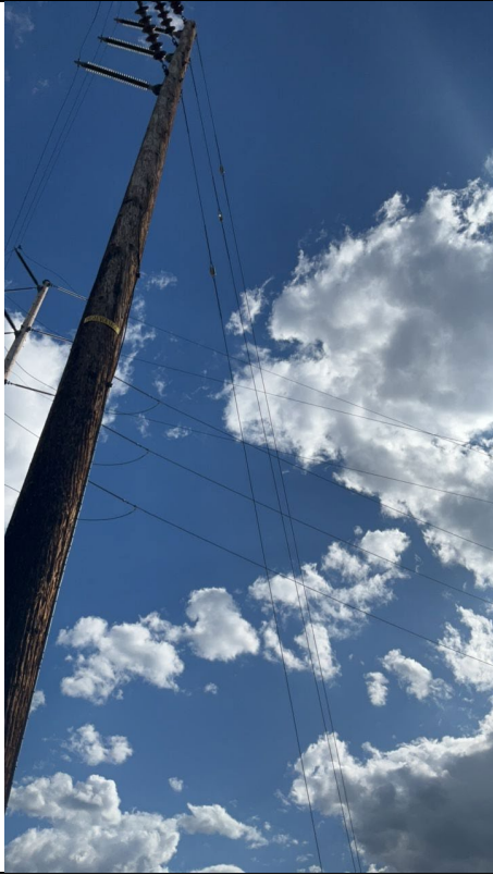
IA1mg1: No covered conductor installed at this location
