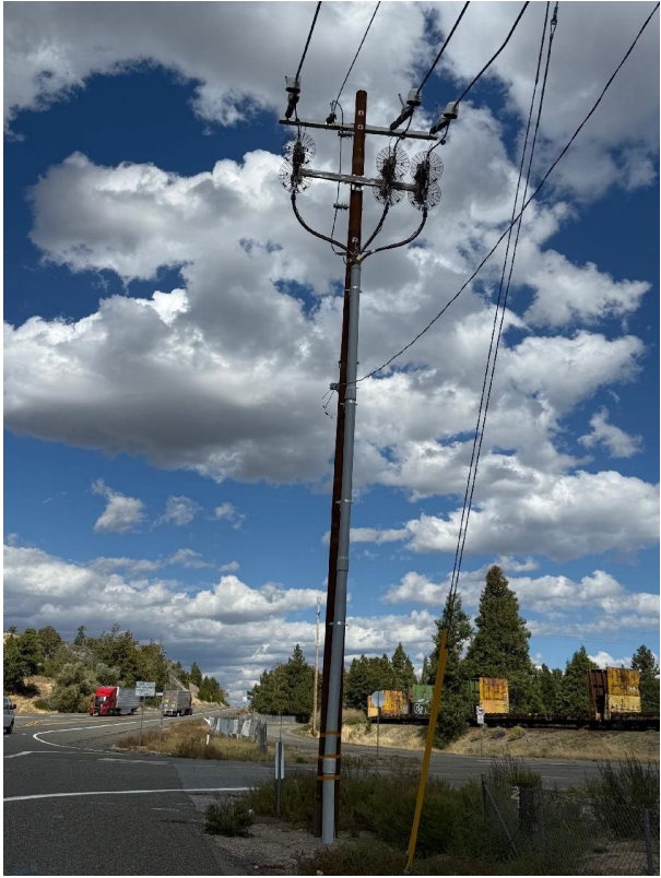
IA1img1: North-facing view showing no overhead and covered conductor installed north of Pole 06241005026600
