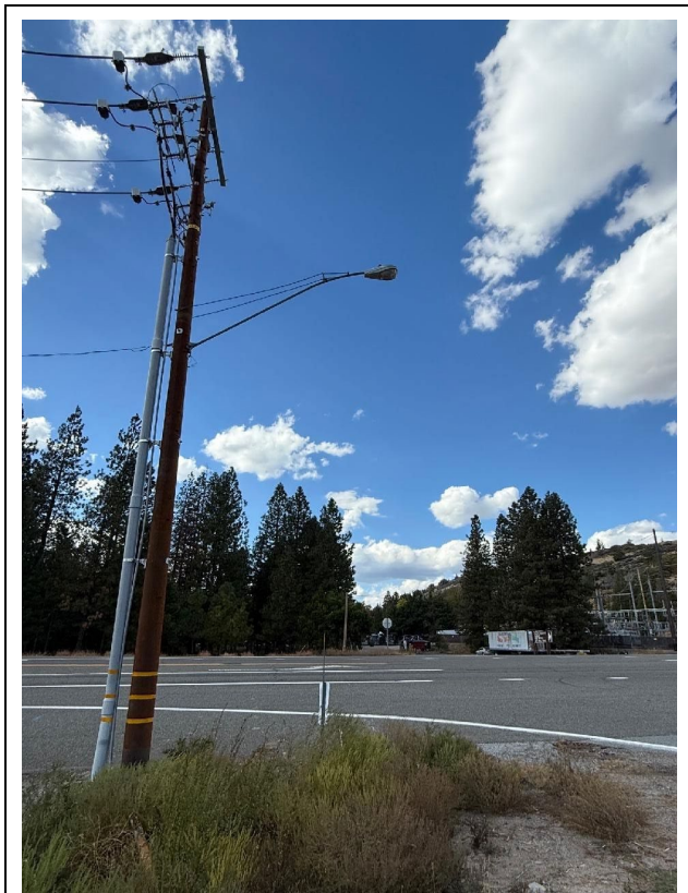
Gimg3: West-facing view showing no covered conductor installed west of Pole 06241005026600
