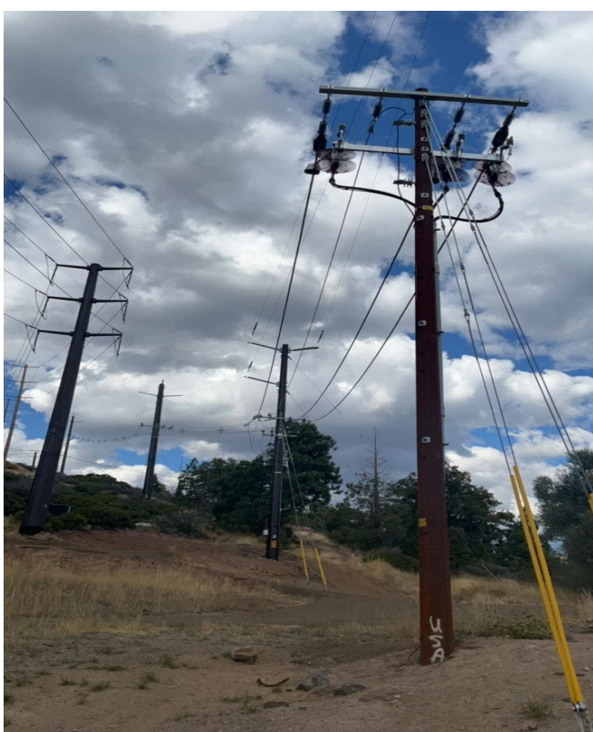
IA1Img1: North-facing view showing no overhead conductor installed south of Pole 06241005026700
