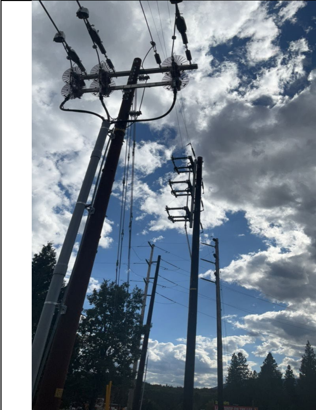
G1mg1: Overall structure, south-facing view with no covered conductor installed south of Pole 06241005026700
