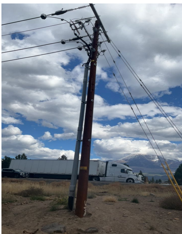
IA1Img2: East-facing view showing riser and no covered conductor installed south of Pole 06241005026700
