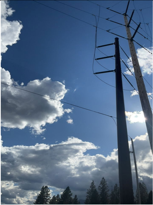
IA1Img1: No covered conductor installed at this location (subject pole shown on the right side of the photo)
