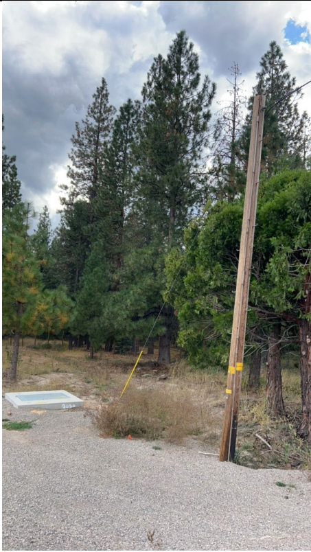
IA1Img1: South-facing view showing no CAL FIRE-approved non-expulsion fuses installed on Pole ID 06241005.025601
