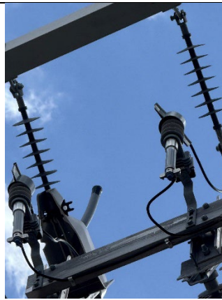
IA1mg2: Surge/Lightning arresters on the other side of the pole
