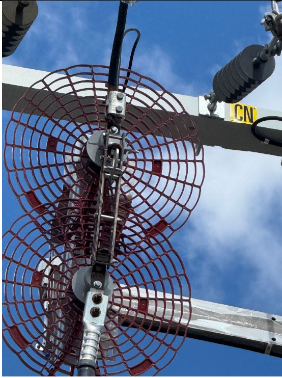
IA1Img3: Disconnect switch
