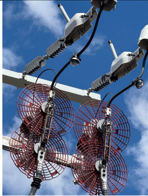
IA1Img4: Disconnect switches
