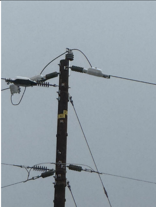
IA1mg1: Close-up view showing no CAL FIRE-approved non-expulsion fuses installed on the pole
