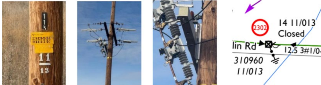
Picture 1: Grid Hardening ID 7112939 at coordinates 41.71135922538462, -122.59285126282776. Picture taken January 29, 2026.
