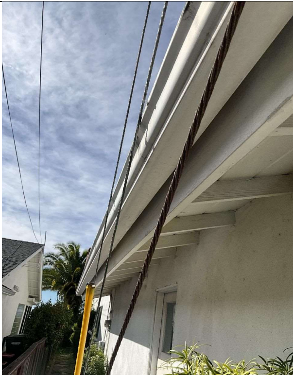
IA1img3: All three down guy wires are rubbing against house gutter
