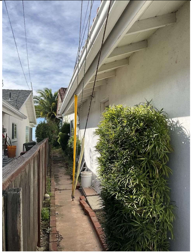
IA1img2: All three down guy wires are rubbing against house gutter
