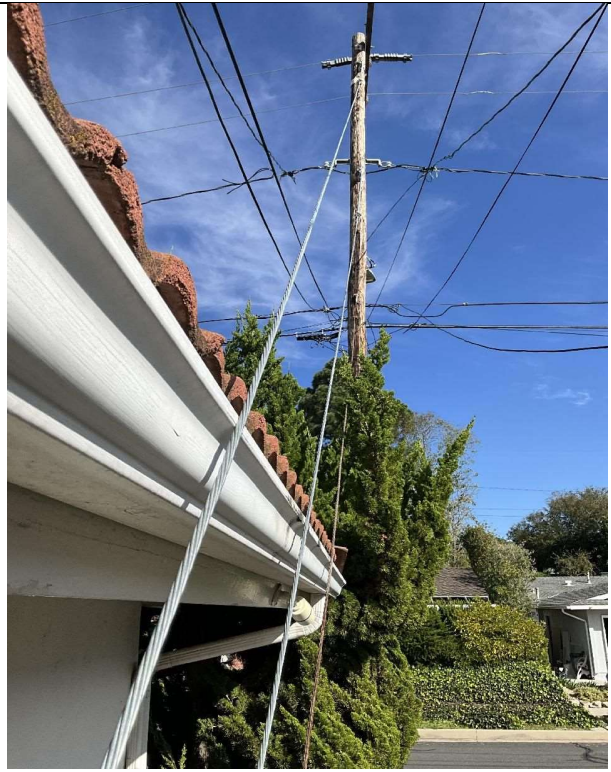
IA1img4: All three down guy wires are rubbing against house gutter
