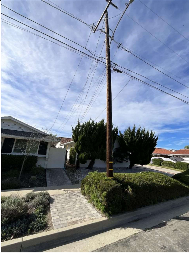
IA1img1: All three down guy wires are rubbing against house gutter
