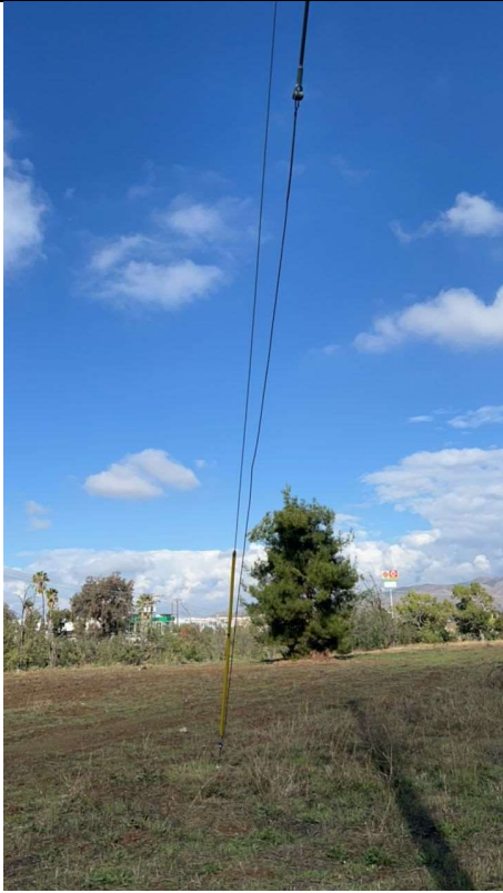
IA1Img1: View showing slack in down guy
