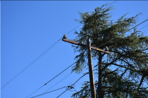
IA1Img3: View of bare conductor
