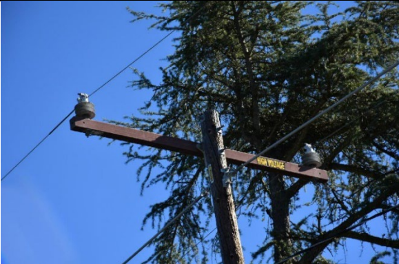
IA1Img4: View of bare conductor
