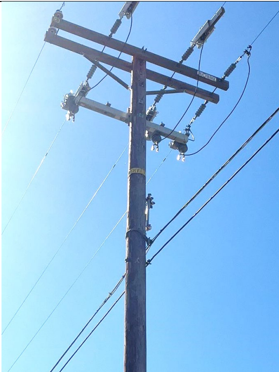
IA11mg1: Three empty cutouts observed.
