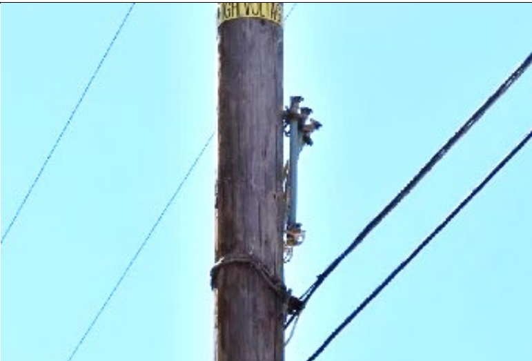
IA11mg2: Three fuses observed hanging from the pole.
