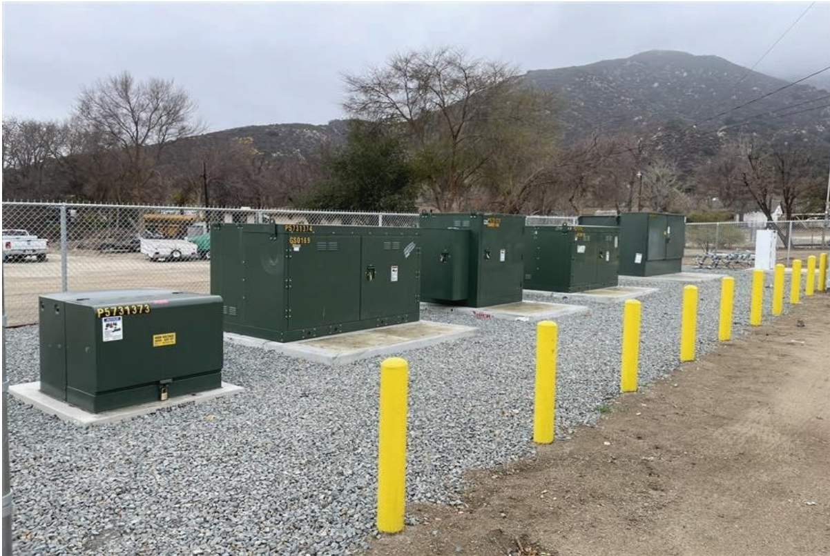
Figure SCE 8-9: Images of Isolation Transformers used for Grounding Conversion
