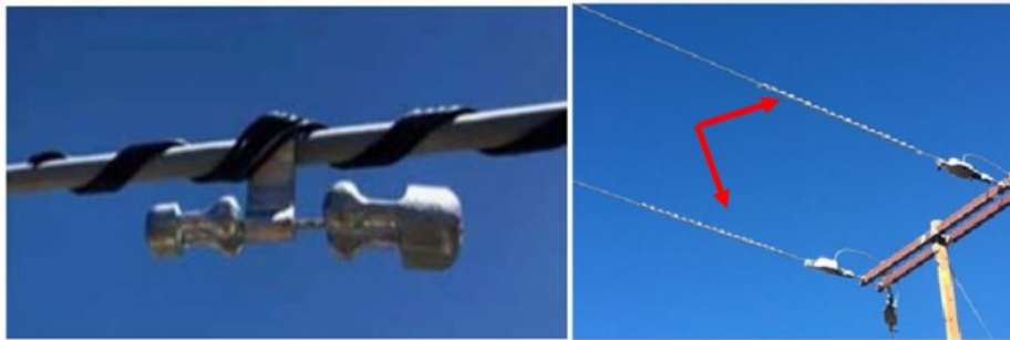
Figure SCE 8-02: Types of Vibration Dampers: Stockbridge Damper (left) and Spiral Damper (right)
