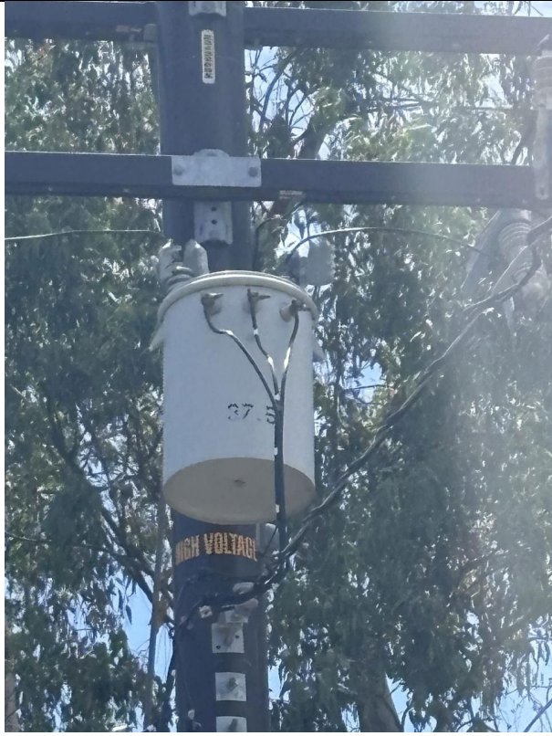
IA1Img1: Transformer bushings unhinged
