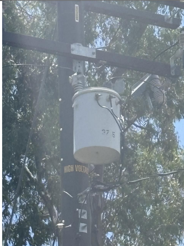
IA1Img3: Transformer bushings unhinged
