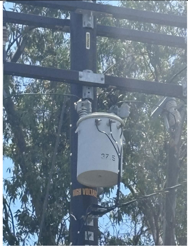
IA1Img2: Transformer bushings unhinged
