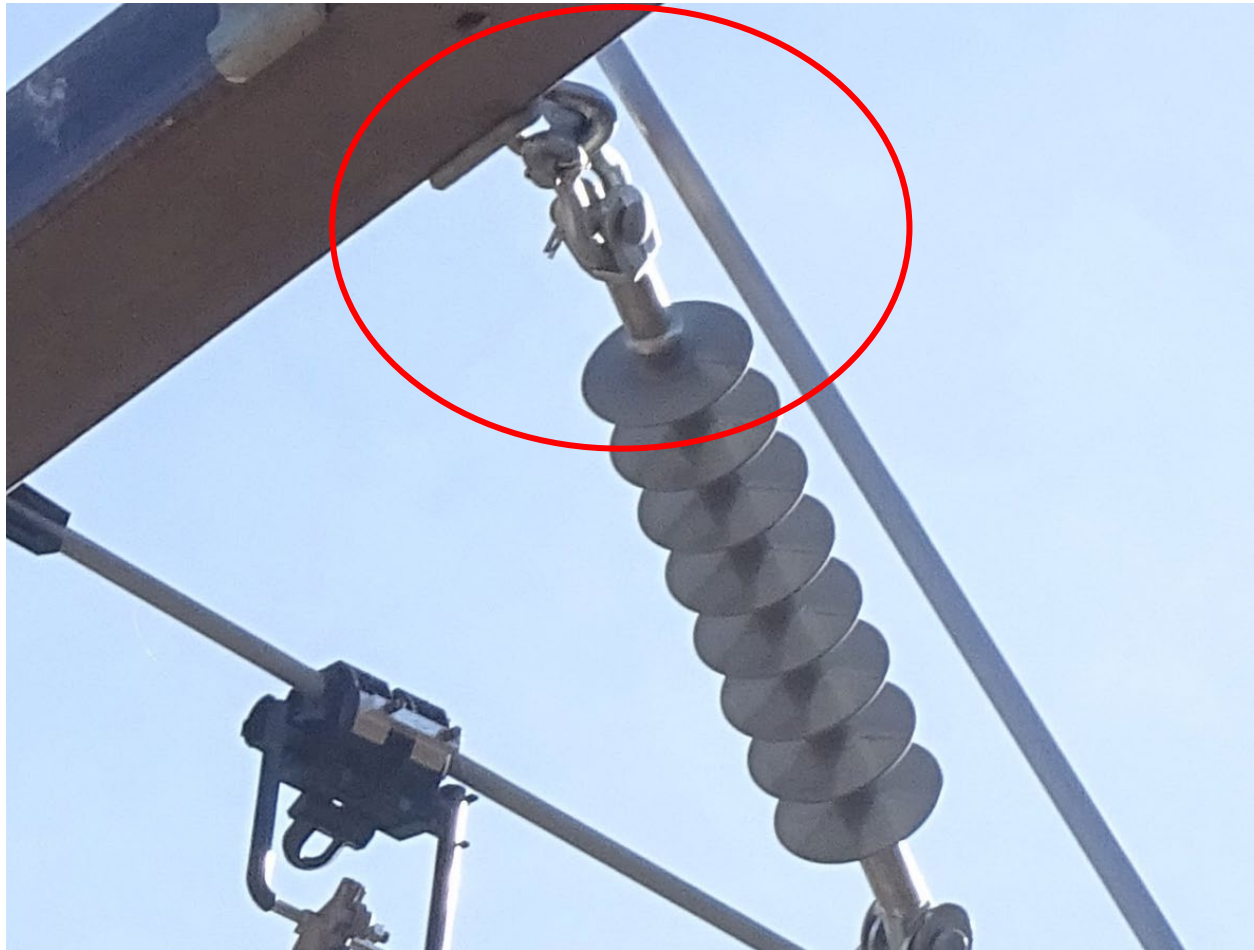
Figure 2 - Image acquired during QA/QC inspection on 12/17/2024 showing clearance between down guy and insulator
