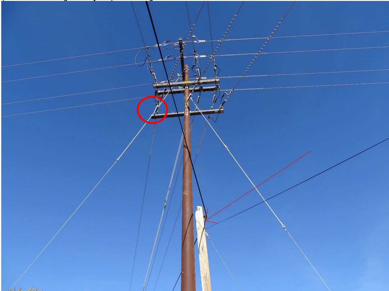
Figure 1 - Image acquired during QA/QC inspection on 12/17/2024, notating state of CIP (attached to adjacent pole) and subject hardware identified in notice of violation
