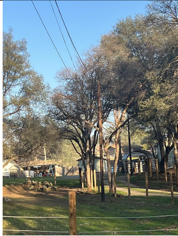
Item1IA1img2: Pole east of 121530972 was observed as a secondary service pole.
