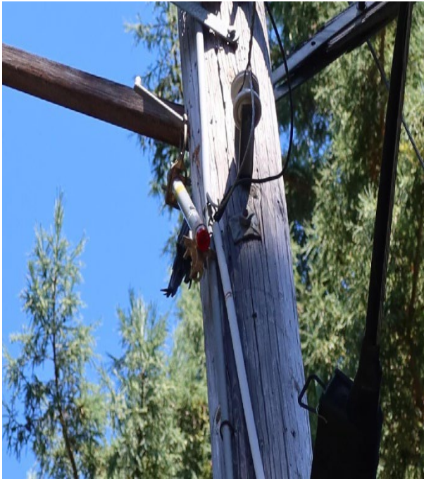
Item1IA1Img3: Hanging CalFIRE-exempt fuse.
