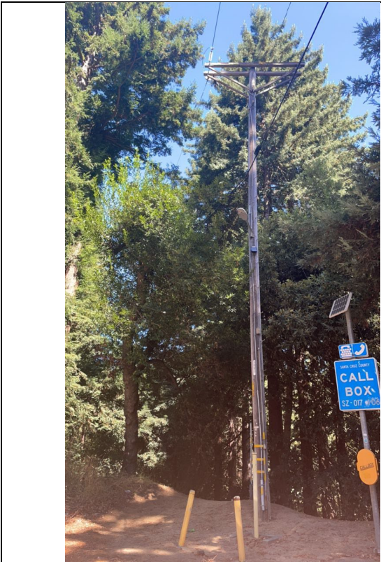
Item1Gimg1: Overall Pole.
