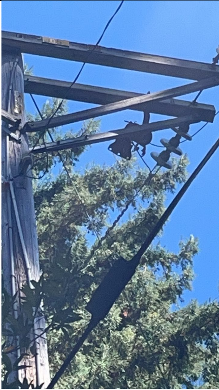
Item1IA1Img1: View of the empty fuse cutout.
