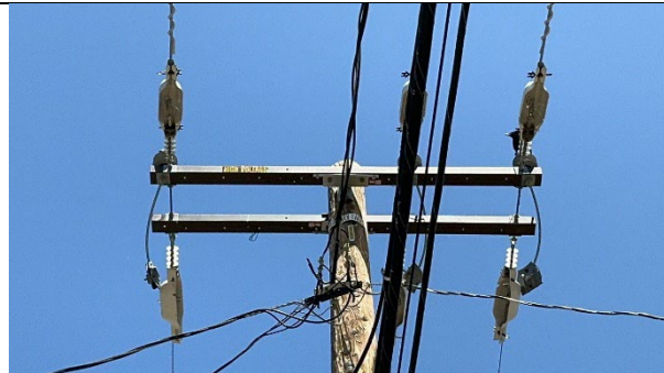
Item1IA1Img4: View showing dead-end wildlife covers seated at approximately ninety degrees.
