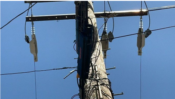
Item1IA1Img3: View showing dead-end wildlife covers seated at approximately ninety degrees.
