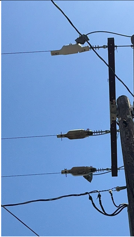
Item1IA1Img1: View showing dead-end wildlife covers seated at approximately ninety degrees.
