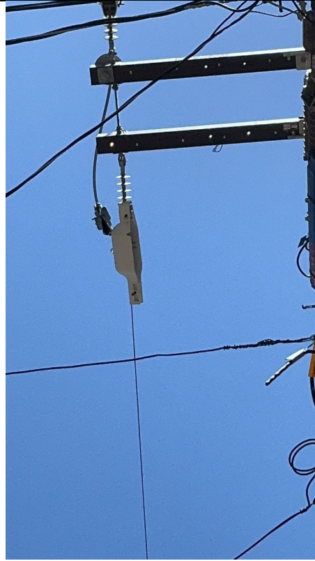
Item1IA1Img2: View showing dead-end wildlife covers seated at approximately ninety degrees.
