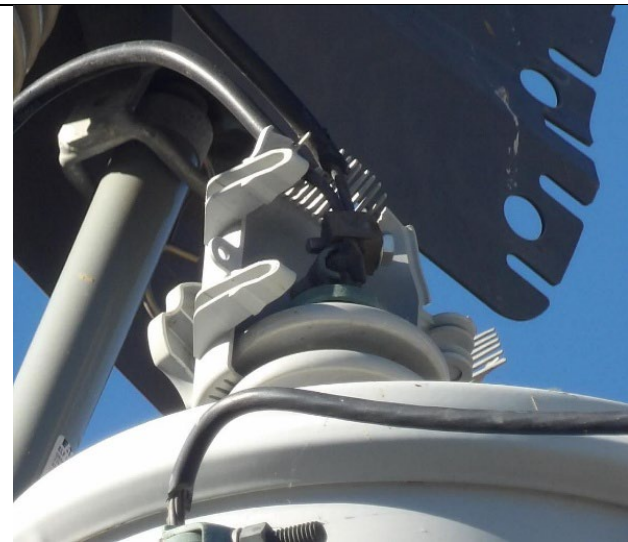
Item1IA1Img3: Close-up view of exposed wildlife bushing cover.
