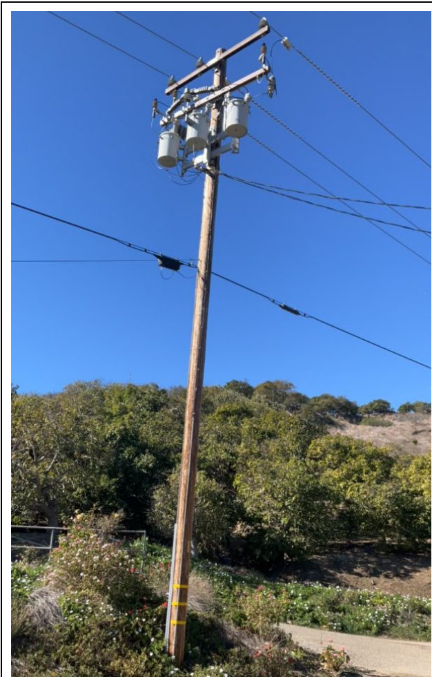
Item1Gimg1: Overall pole.
