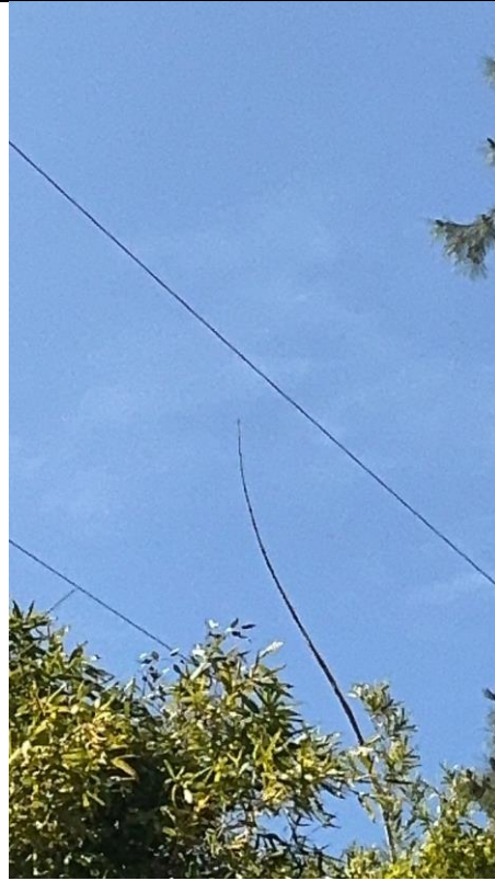
ItemV3: Closer view of the bamboo within 2 feet of the conductor.
