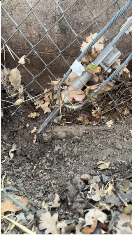
Item1IA1img1: Observed buried guy anchor below grade.
