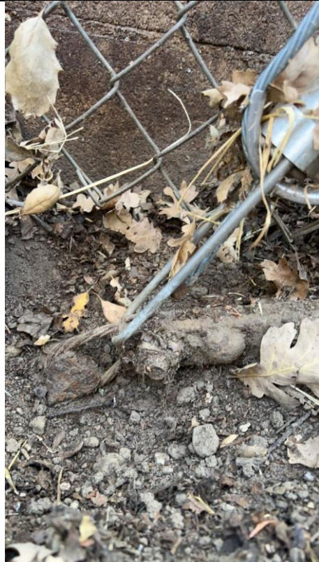
Item1IA1img2: Down guy wire preform is connected to an automatic and not directly to the down guy anchor eye. The automatic is connected to an existing severed down guy loop fastened together by a three-bolt clamp.
