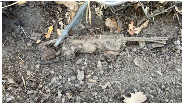
Item1IA1img4: Severed pre-existing down guy loop fastened by a three-bolt clamp.
