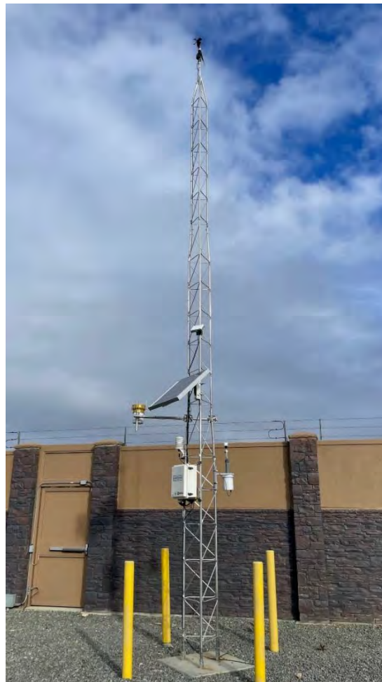
Figure HWT 8.3.2- 2. Weather Station
