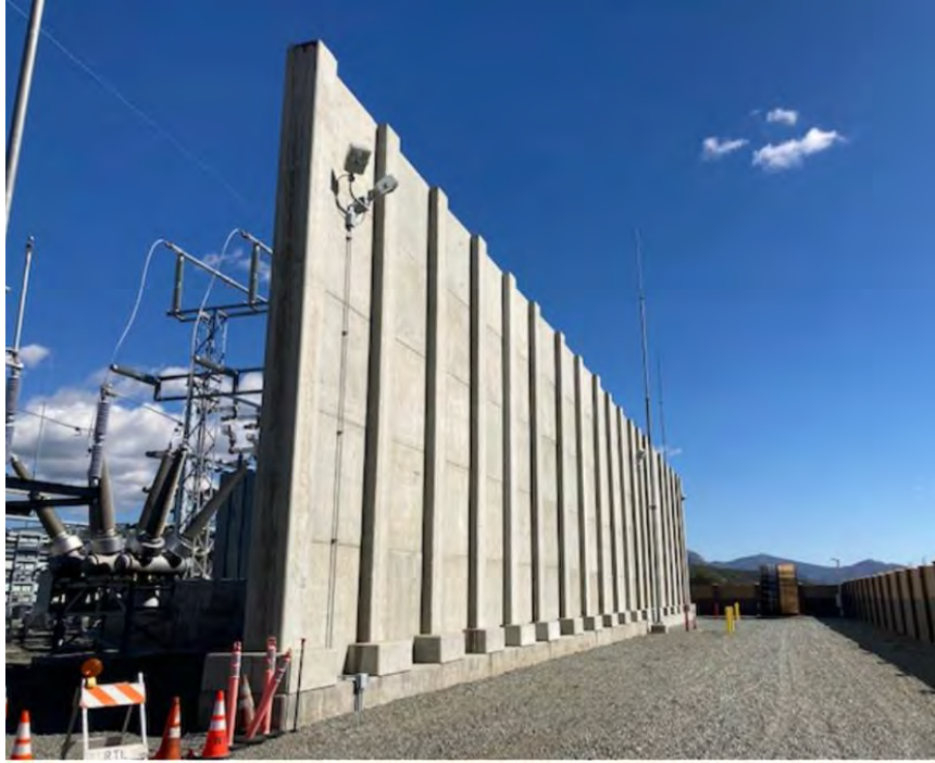
Figure HWT 8.1.2- 1. Transformer Fire Barrier Wall
