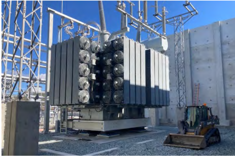
Figure HWT 8.1.2- 3. Transformer Seismic Isolation Pad
