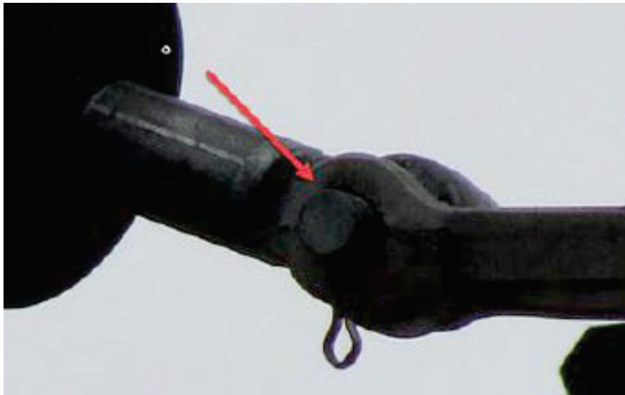
Figure A: Cotter pin improperly secured
