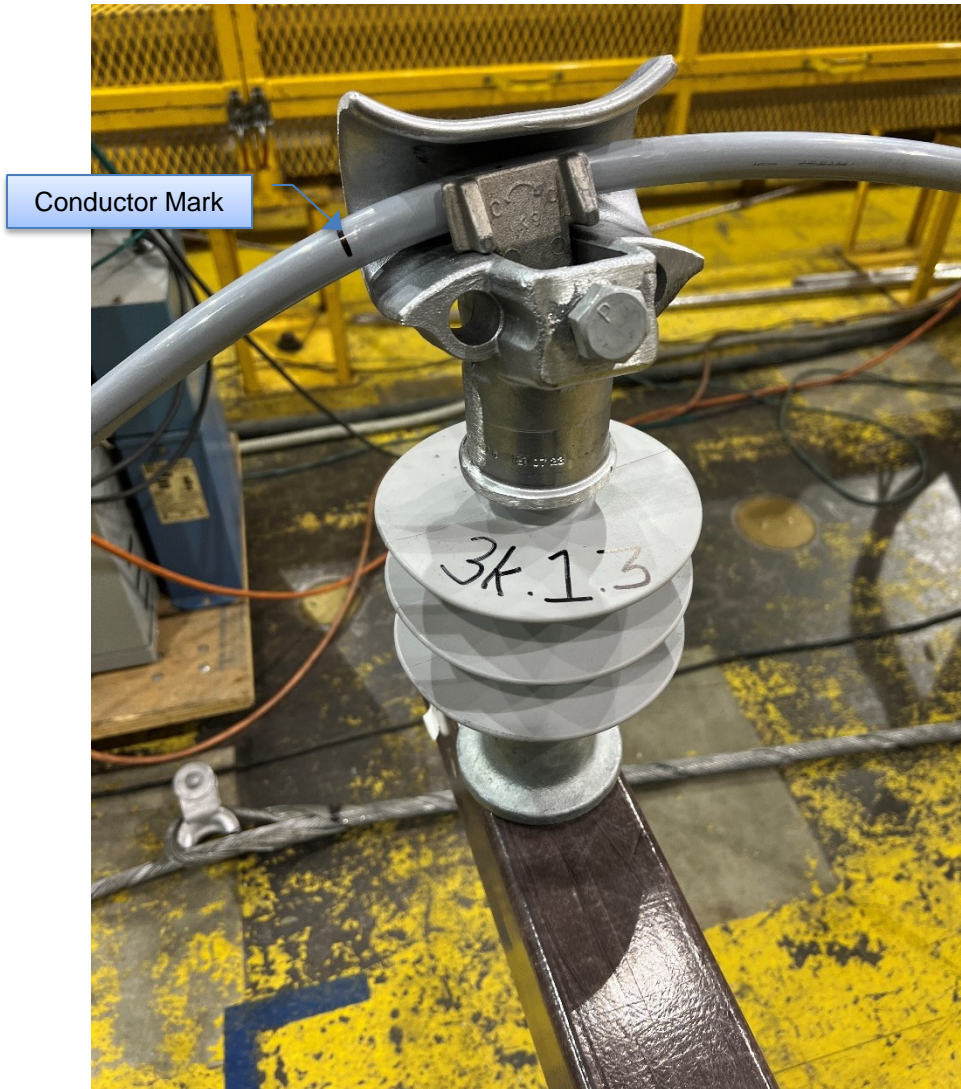
Figure 6-29: Sample 3K.1. – Insulator and Cross-arm Condition after Test
