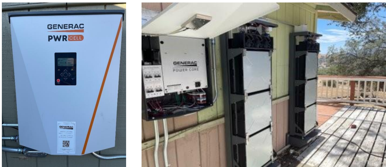
Figure 8-6: FPB Installation at Mobile Home Park Community
