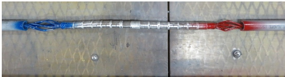
Figure 3-3: ██████ installed on 35 kV 1/0 AWG, 6/1 ACSR
