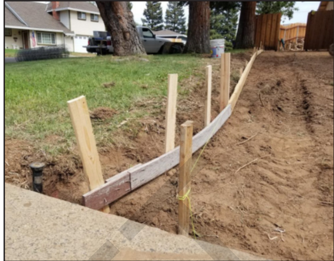
Closeup of new driveway excavation performed by C-8 Concrete specialty contractor. From Investigation 21SA01473
