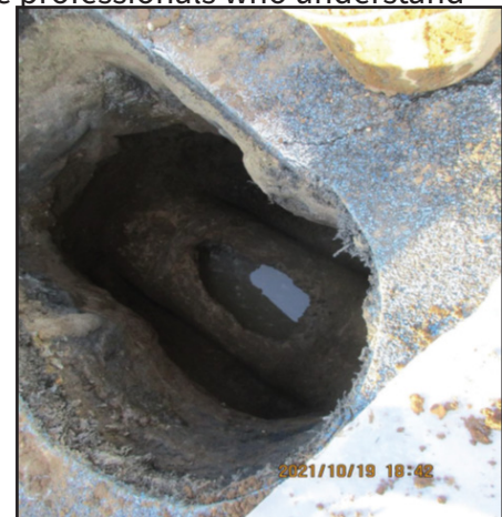
Irrigation pipeline damaged by a D-03 Awnings licensed contractor. From Investigation 21LA01483.
