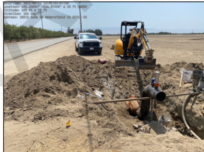
Repair of leaking concrete pipe outside of Bakersfield. Image provided by pipeline operator. From Investigation 21LA01474.
