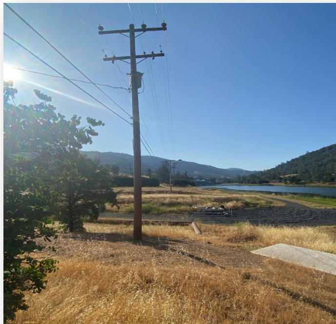
Figure 10 – Distribution PRC § 4292 Pole
